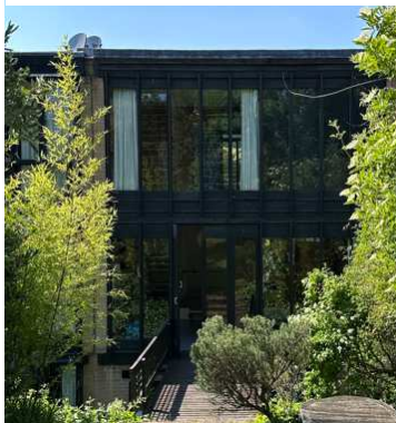
Figure 3 - 2024 Site photo with later painted boards and over cladding at the eaves
