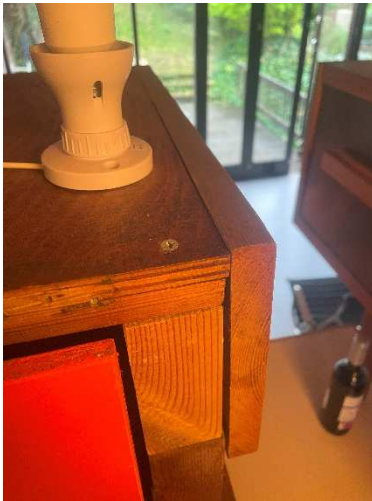
Figure 14 - Poor carpentry to end cupboard with fridge (to be adapted in proposals)
