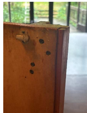
Figure 11 - Hidden screw fixings no aligned inside cupboards
