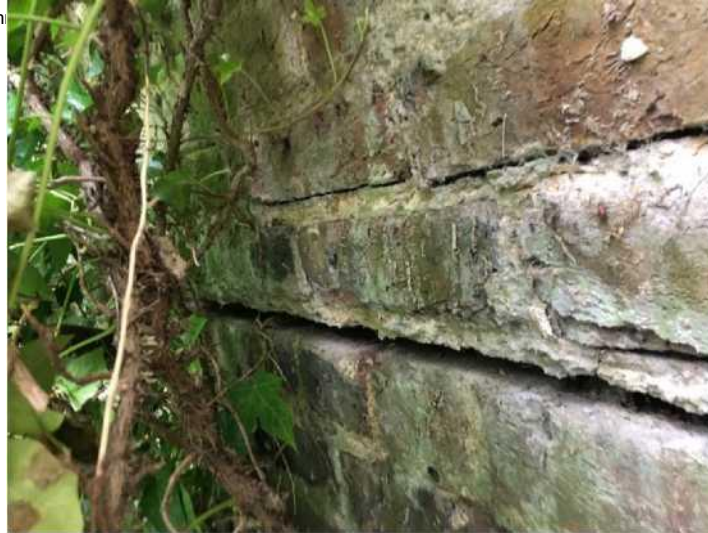
Fig 5. Horizontal open joint, crack and displacement within 3m of the rear
