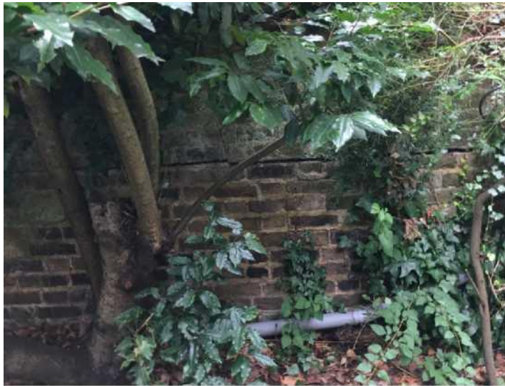
Fig 3. Horizontal open joint adjacent to tree. Note redundant rainwater pipe at low level from balcony outlet.
