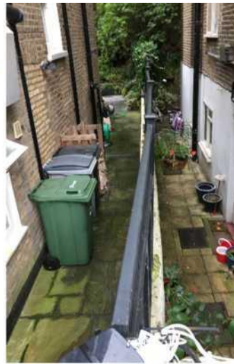
Fig.12 Wall between 10 and 12 - viewed from above the wall facing No.58 towards the rear with No. 12 to the left and No. 10 to the right.
