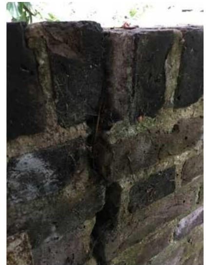
Fig 4. Vertical crack and displacement to wall approx. 3.5m from the rear boundary.
