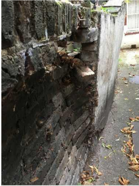
Fig 9. Wall between No. 10 and 58, viewed from the No. 58 side facing the junction with No. 12. Blown brickwork and rendered section of wall beyond.
