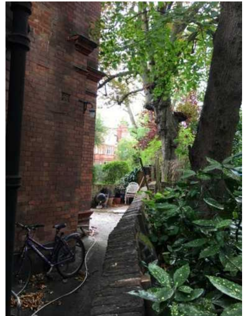
Fig 10. Wall between No. 10 and 58, viewed facing No. 8 with No. 58 to the left. Leaning and curved wall adjacent to the mature tree.
