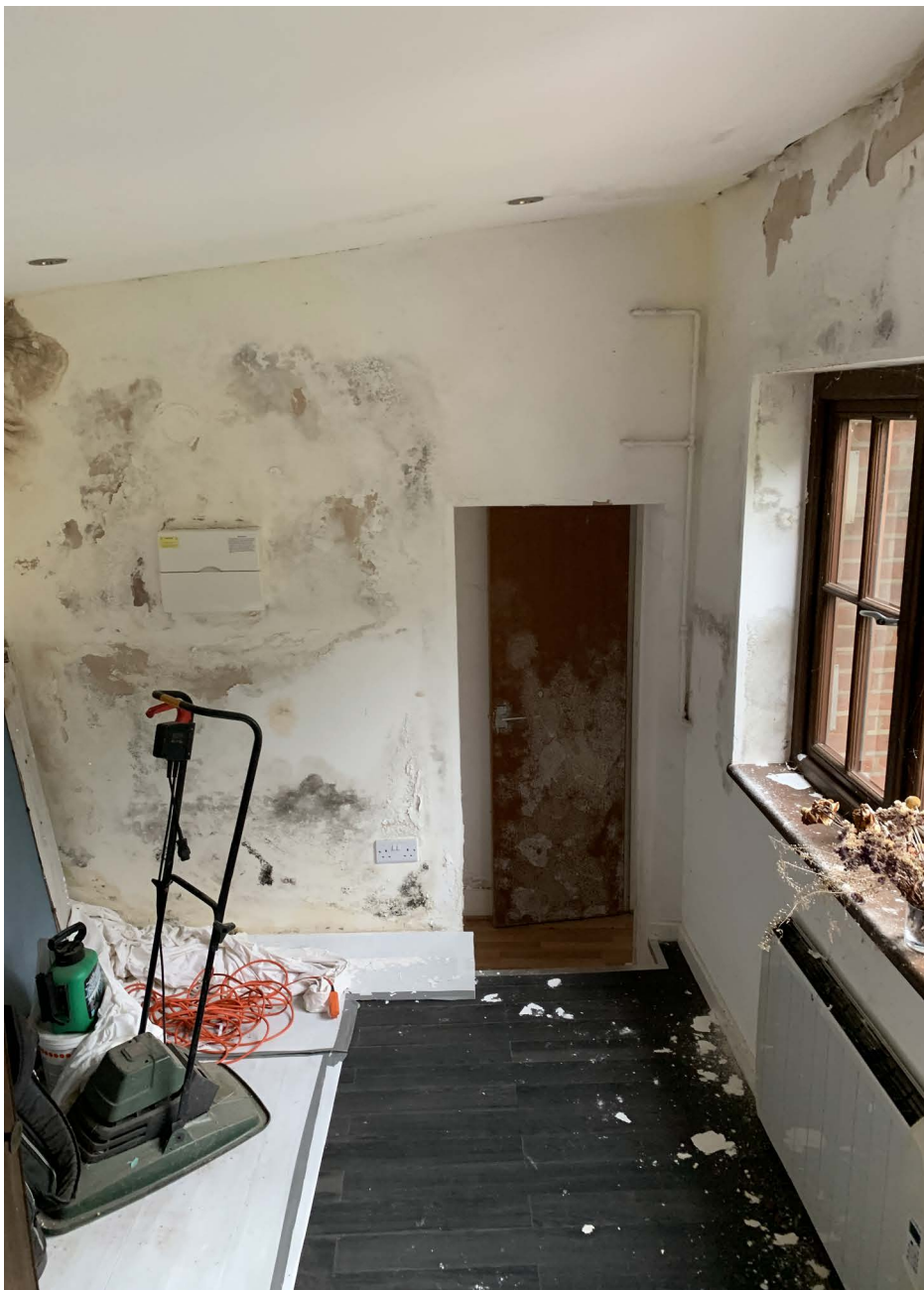
Figure 14 Photograph showing internal damage in the garden studio outbuilding caused by the leaking roof.
