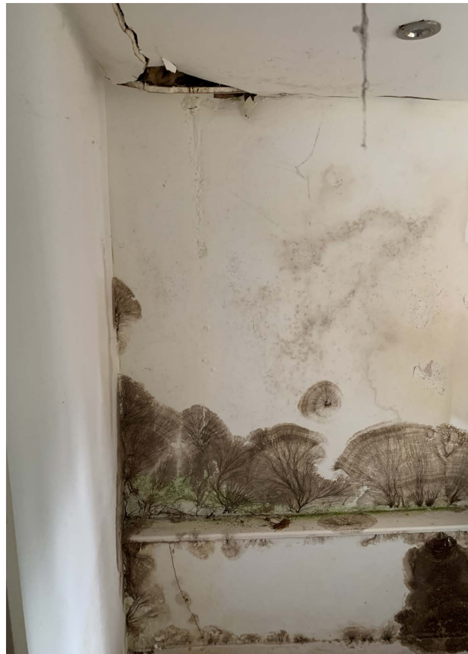
Figure 15 Photograph showing internal damage in the garden studio outbuilding caused by the leaking roof.
