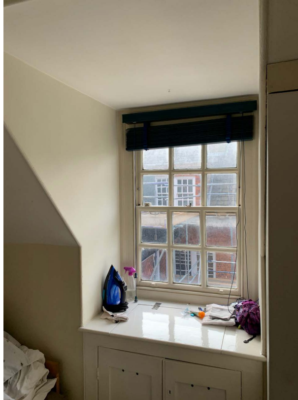
Figure 17 Photograph of the existing side (South-East) elevation sliding sash window as seen from inside.
