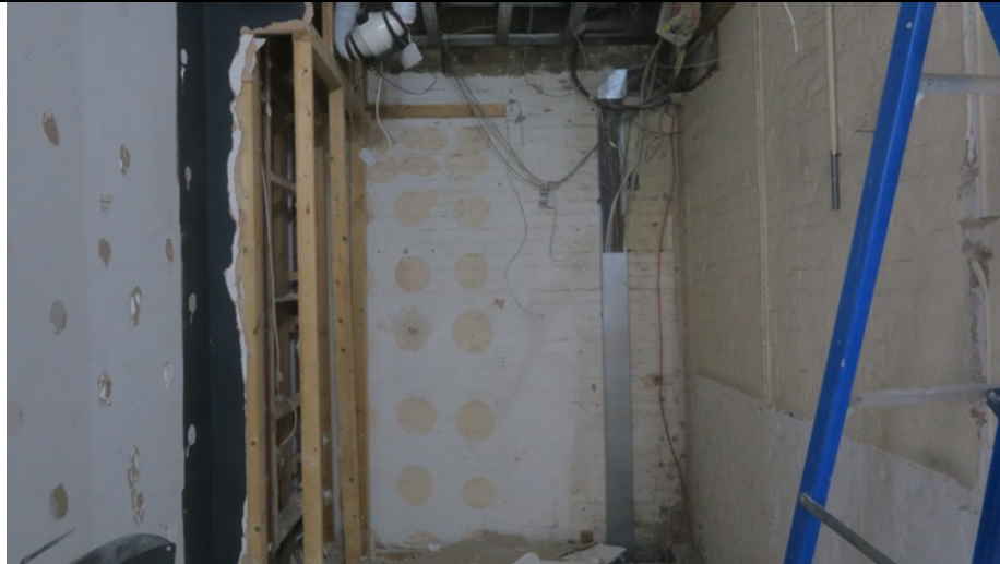
1 st floor to No.25 Neal Street former changing room area with retained painted finish.
