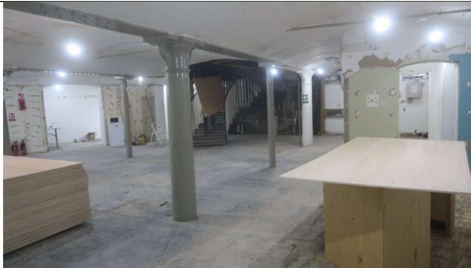
Cellar area to No.25 Neal Street retail unit with painted finish retained.
