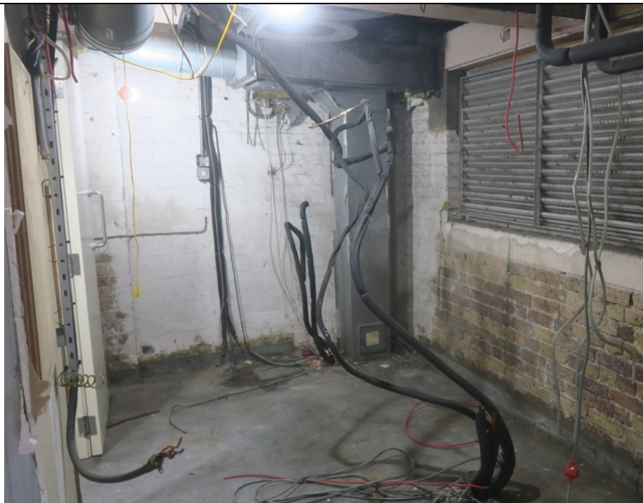
1 st floor to No.25 Neal Street former service riser / staff area with retained painted finish.
