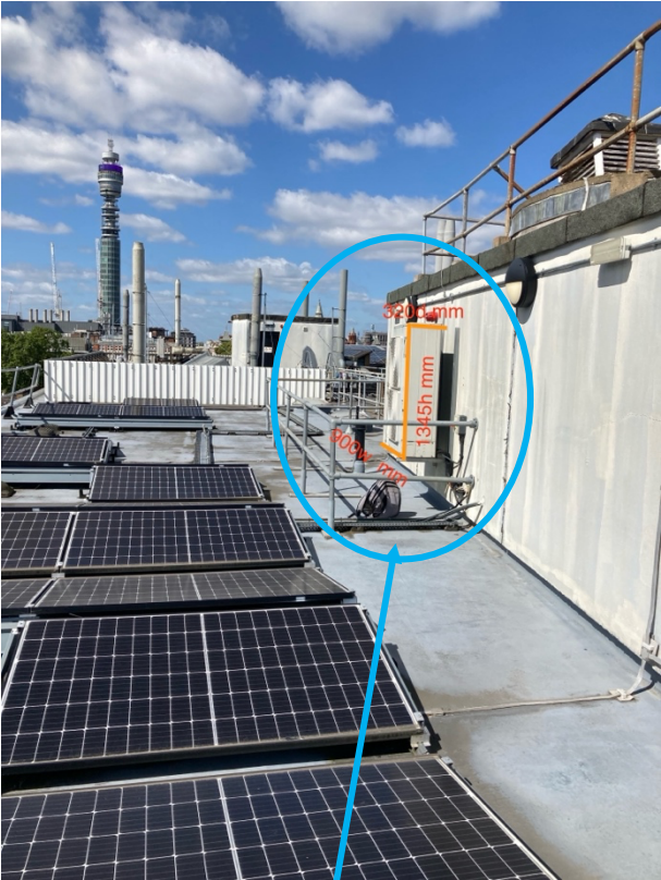
Existing redundant condenser unit to be removed along with associated refrigerant pipework
