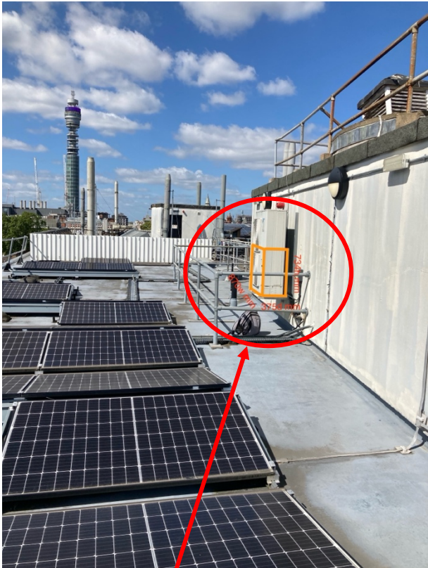
Proposed Condenser Unit to be installed in the same location supported off the wall on new Gallow Brackets with new pipework to follow the route of the existing
