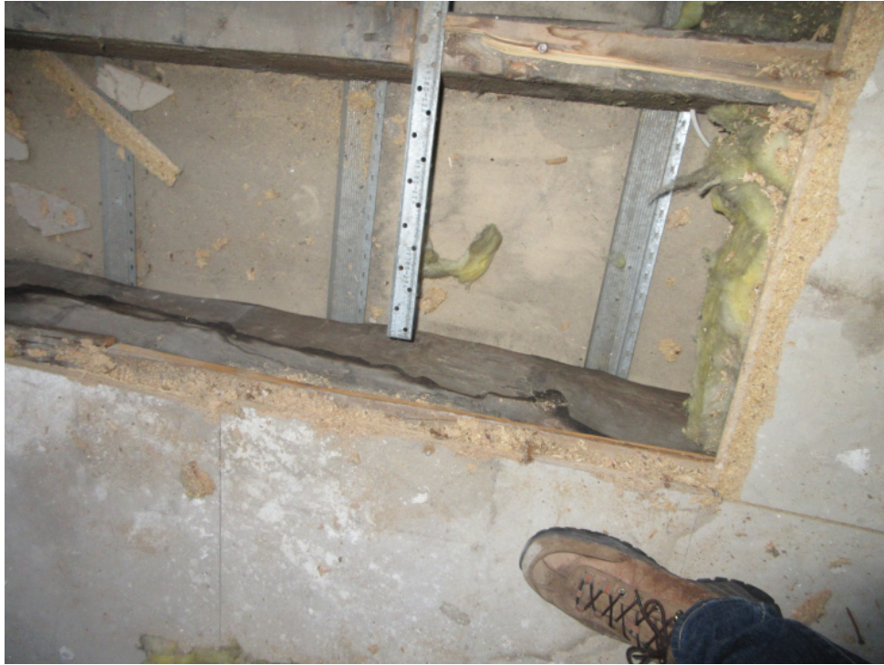
Another non regularised joist.
