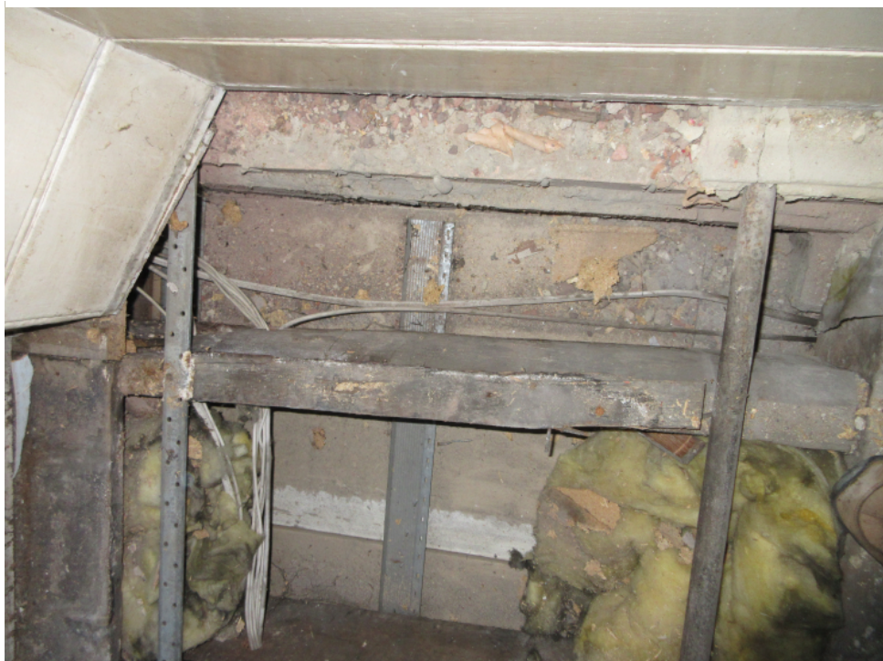
Tie bar and galvanised strap at front wall.
