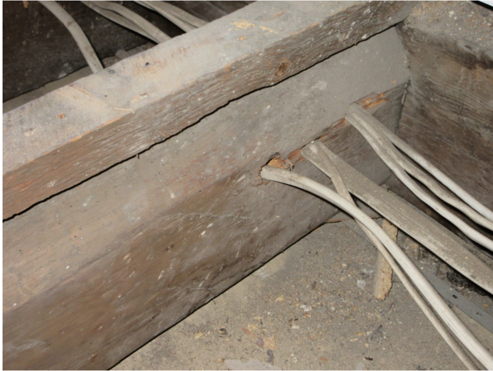
A number of timbers not regularised.
