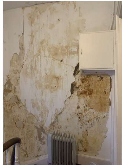
Internal damage from roof leaks
