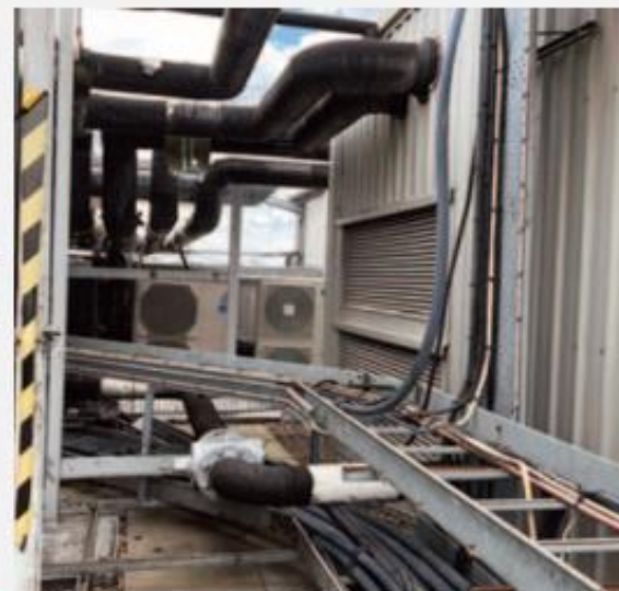
Figure 12: Lifts and plant machinery will be removed; specialist M&E consultants and engineers should be consulted regarding re-use potential.
