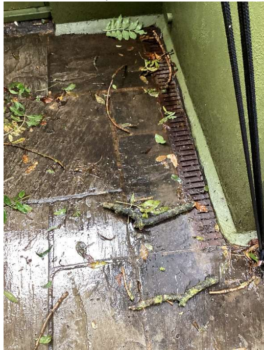
4 Debris in courtyard
