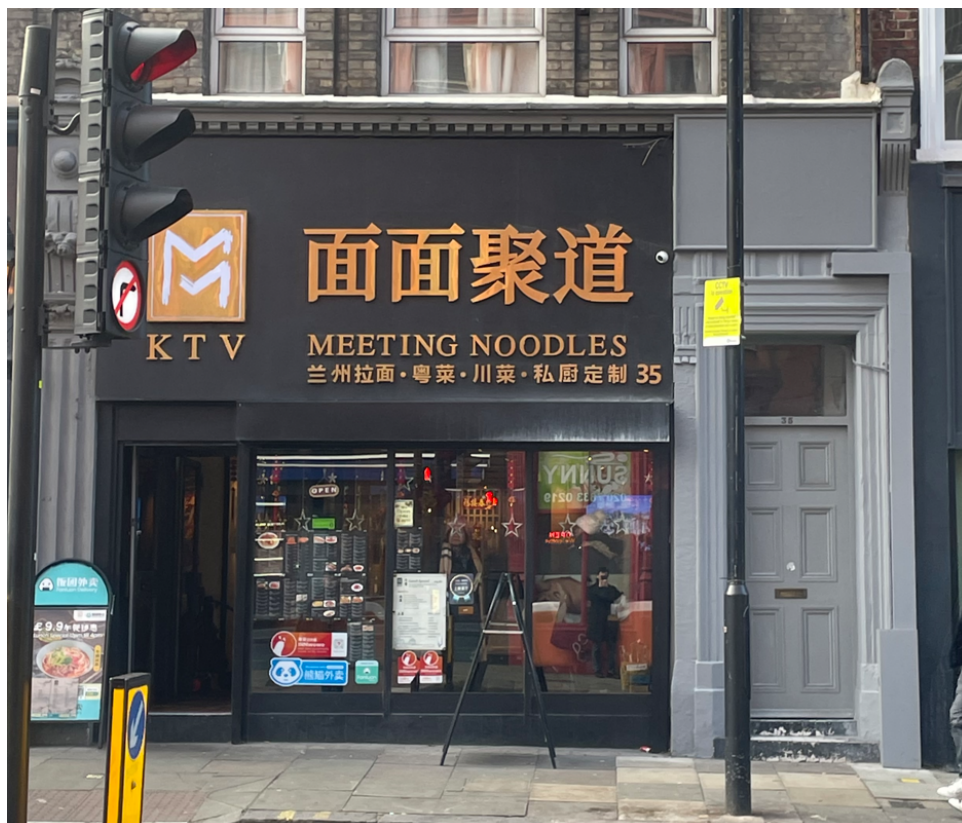
2. Front elevation of site with gas riser installed (to right of grey doorway)
