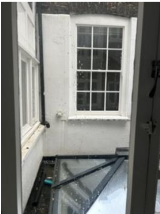
Figure 1: Photo provided by the applicant looking from the rear ground floor room across the lightwell towards the front the property.
