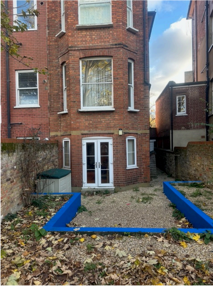
Views of rear of 37A Adamson Rd Garden currently has minimal planting and is gravel.
