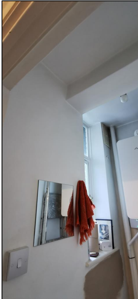
Photo 8: Downstand above toilet room in line with external wall of inset balcony
