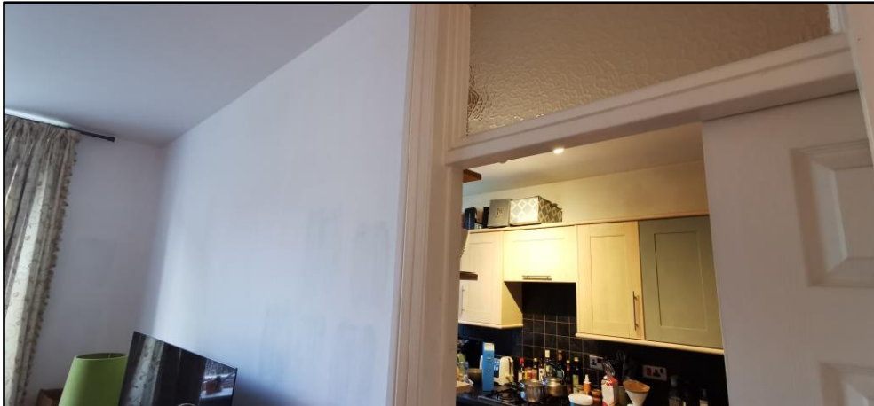
Photo 10: Wall between kitchen and living room with full height opening proposed to be demolished
