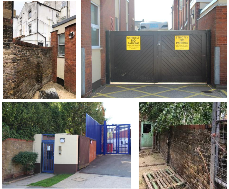
(top left) Image of boundary wall on the west side of the Stables building (top right) Image of vehicle gate from outside (Fortune Green Road) (bottom left) Image of pedestrian gate from outside (Hillfield Road) (bottom right) Image of western boundary wall
