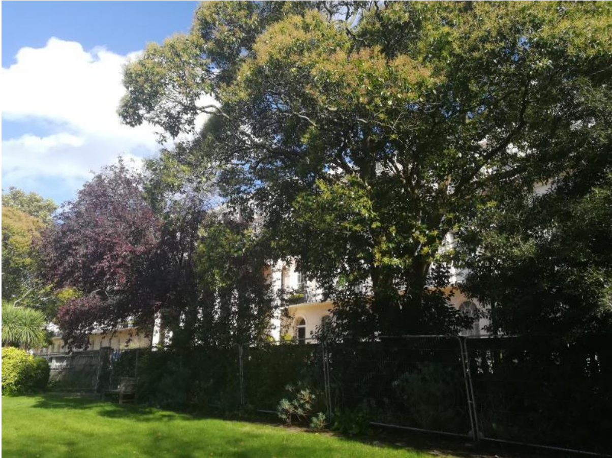
Figure 4: Looking north-east towards the eastern retaining wall that has been fenced-off, showing T491 (front centre-right) as a point of reference.
