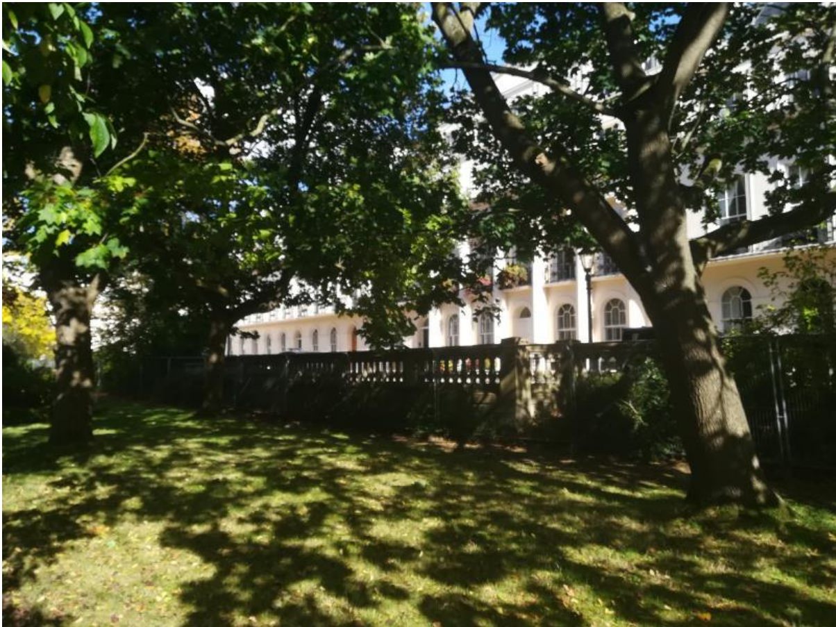
Figure 3: Looking north-east towards the eastern retaining wall between T221 (front right) and T222 (front left), showing its typical detail that is broadly consistent throughout.
