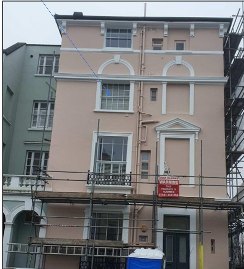
Street view of 33 Regent's Park Road showing the non matching glazing bars to the second floor sash window
