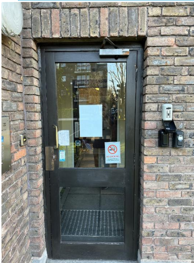
Front Entrance Door
