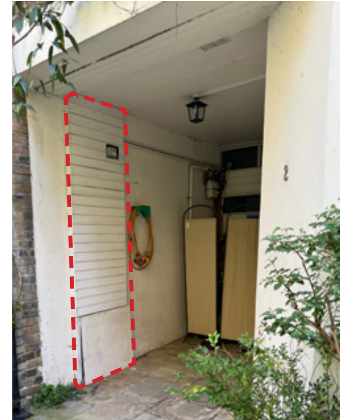
To be removed, electricity boxes concealed in joinery
