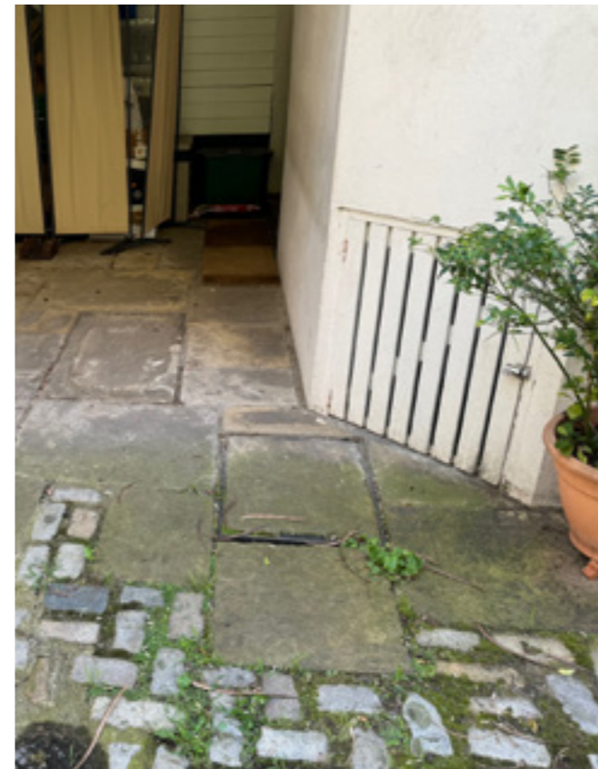
Hatch to be retained, door replaced with a flush panel. Position of manhole retained.
