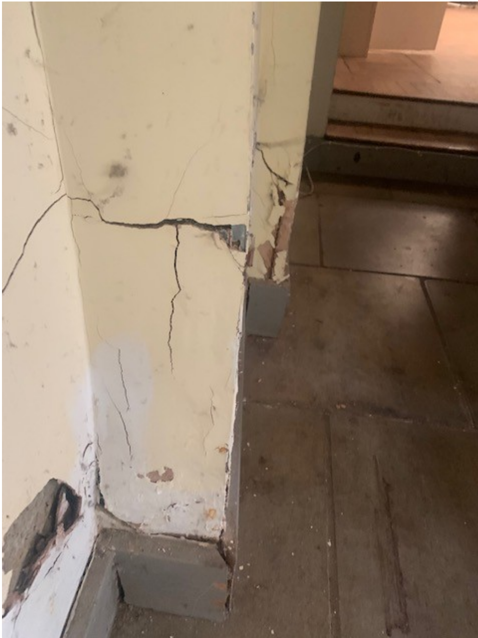
side view on damage to external boundary wall
