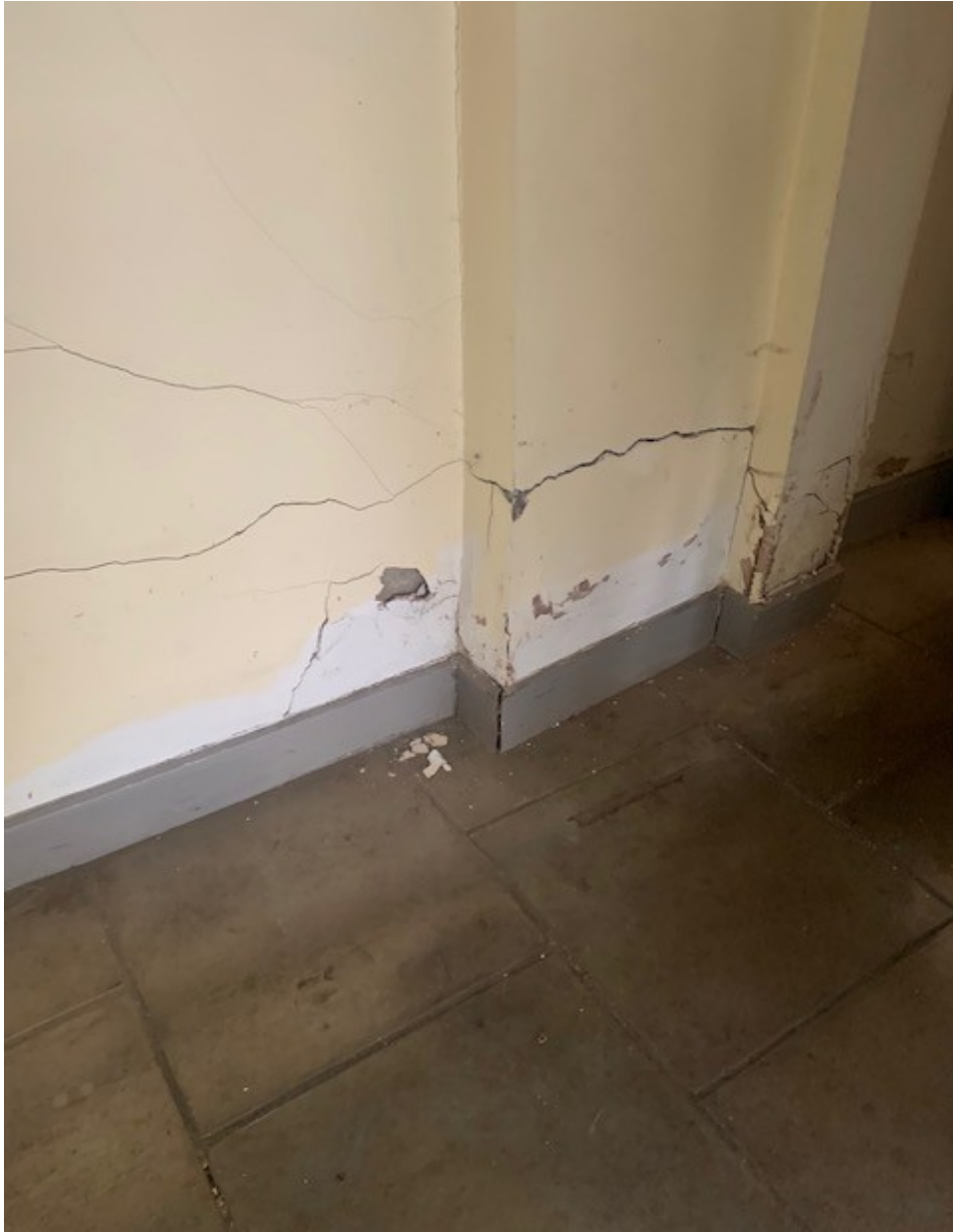
Damage to the external boundary wall
