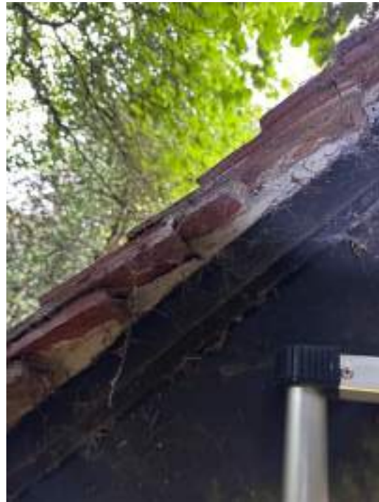
Inadequate lap on tile coursing
