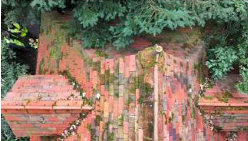
Photograph from UAV / drone showing missing finial from east end of ridge.
