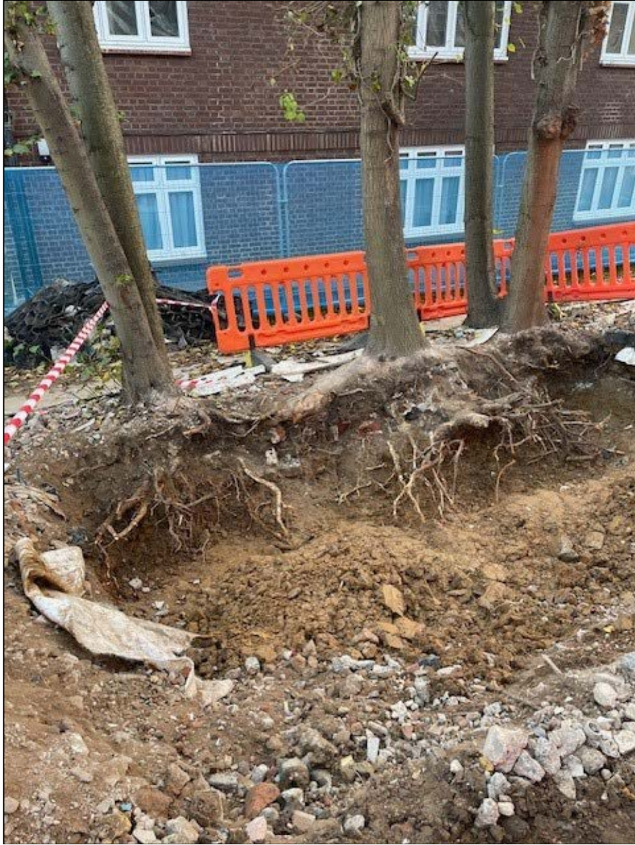
Photograph 3: Damaged roots to all limes on neighbouring property
