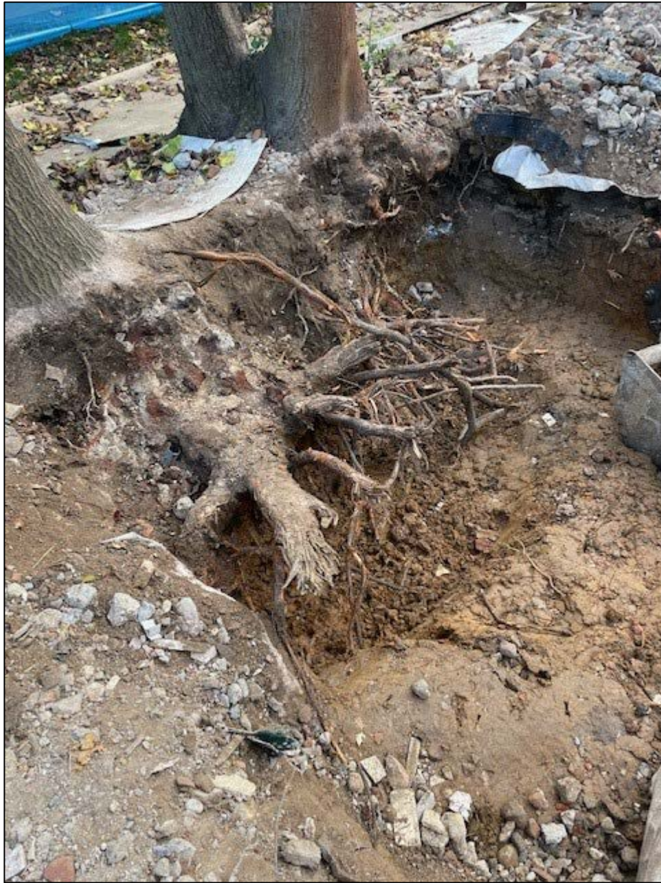
Photograph 1: Example of damaged roots uncovered
