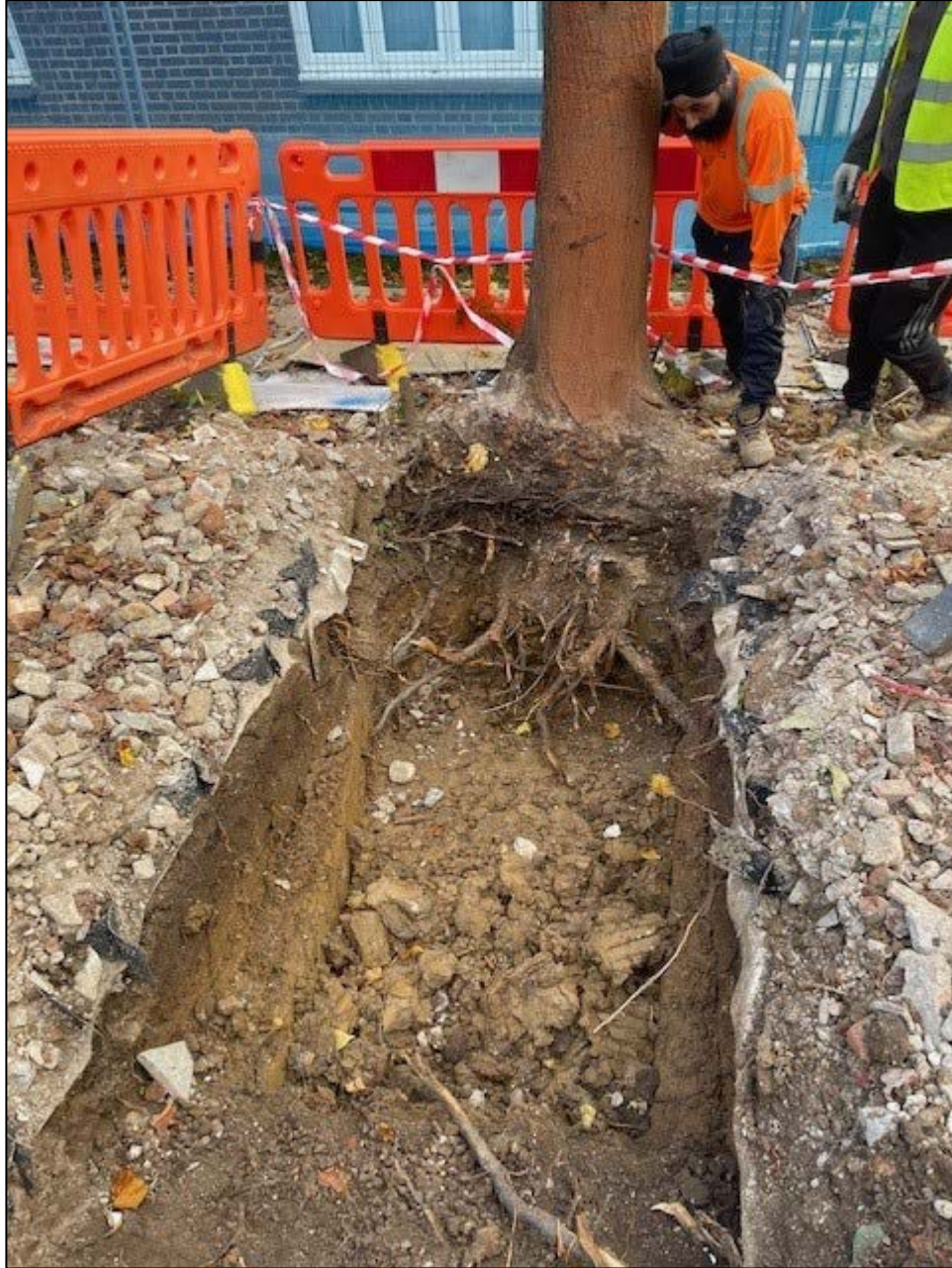
Photograph 2: Further damaged roots
