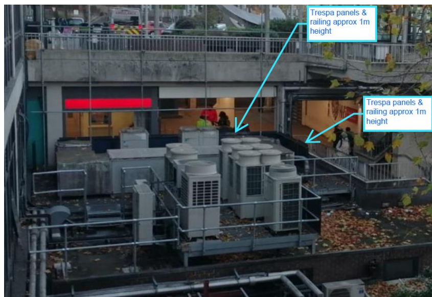
Image 3. Existing railing: trespa panel railing to be remove to facilitate the installation of the new fencing
