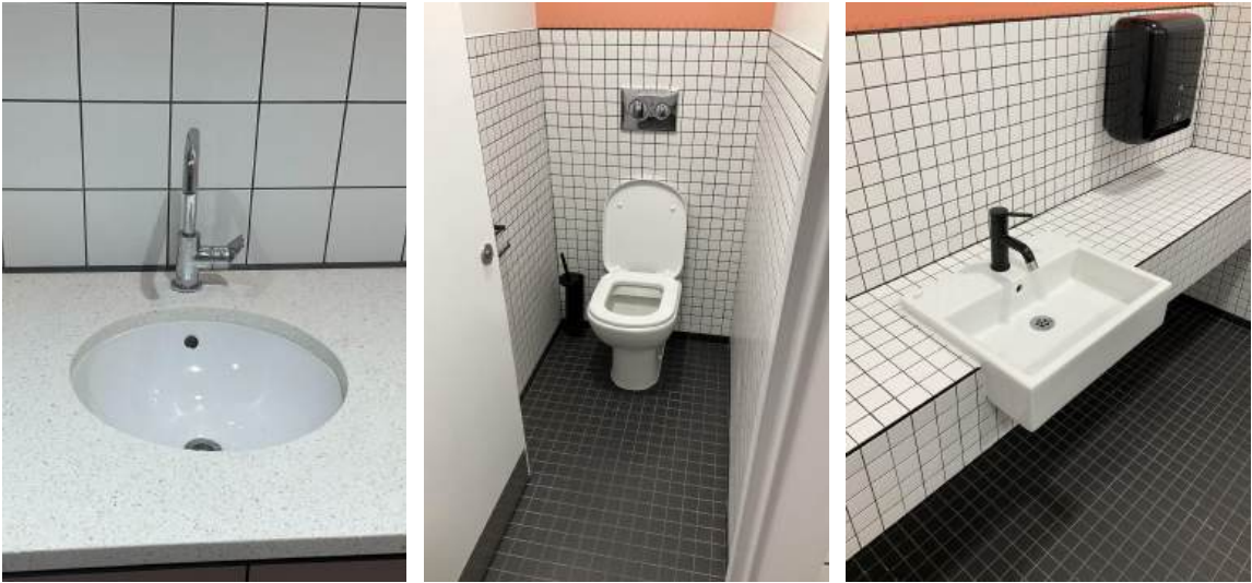
Various sanitaryware types across 125 Shaftesbury Avenue.
