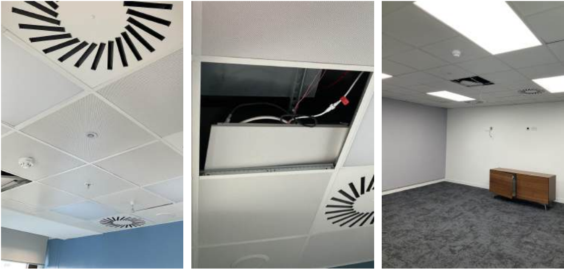
Examples of ceiling grid systems with integrated lighting and detectors.
