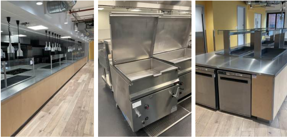
Commercial kitchen equipment across Level 2.
