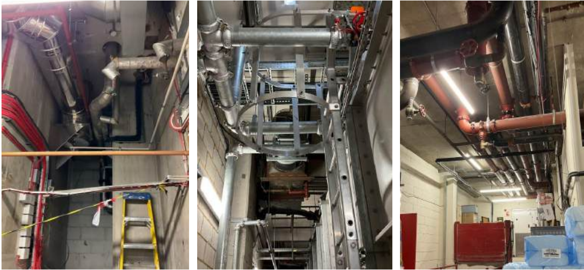
Various MEP plant equipment
