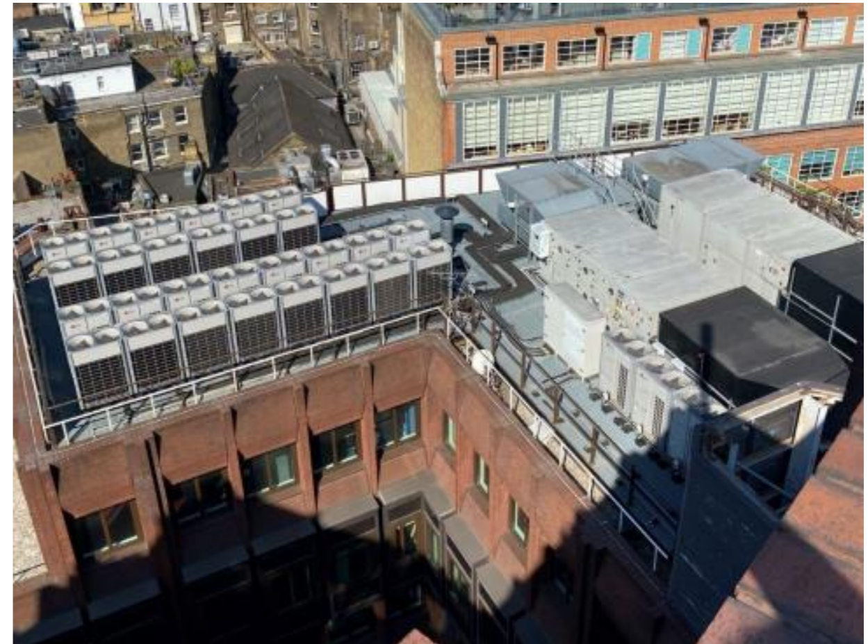
Figure 2.4.4: photograph showing external VRF and AHUs at roof level (L07), demonstrating the condensed and constrained spatial arrangements at roof levels with the current plant equipment and arrangements.
