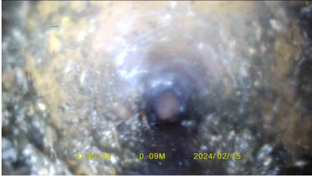
7d9258fa-146f-4850-be93-c5bf5397d76f.jpg, 00:00:10, 0.09 m Settled deposits, fine, 20% cross-sectional area loss, start
