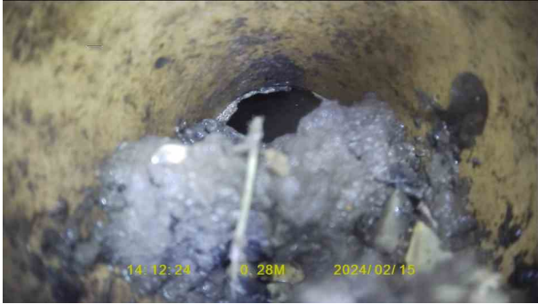
0b747a0b-873a-46c3-b4fc-464612ea82f8.jpg, 00:00:22, 0.28 m Settled deposits, fine, 75% cross-sectional area loss
