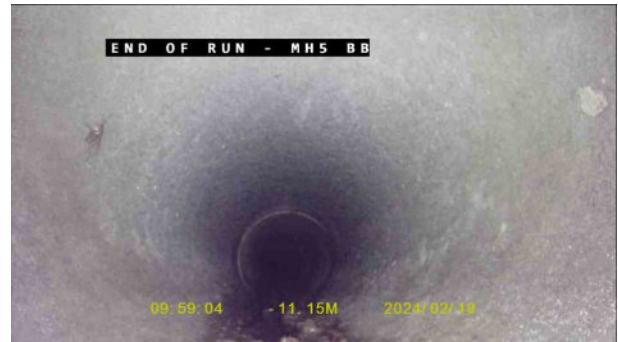
5594bd12-d4fa-41d8-b5f4-3b3c3d60c35d.jpg, 00:01:19, 11.15 m Finish node, manhole, reference: MH5 Branch B
