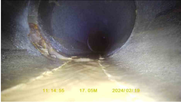
26c73e70-8711-4829-a15d-ed0453455f97.jpg, 00:03:02, 17.05 m Joint displaced, medium
