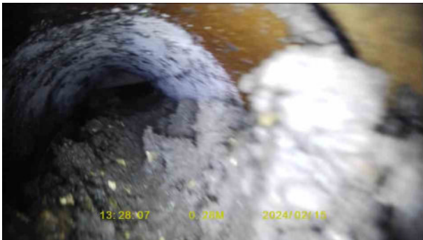
506d008a-a4ca-4920-9f11-68f6314c14b6.jpg, 00:00:21, 0.29 m Joint displaced, medium
