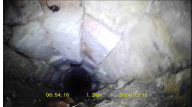
6dfa7ba2-8ce3-4a62-89f8-06e017bbc96c.jpg, 00:00:32, 1.24 m Displaced bricks, single brick false from 10 o'clock to 3 o'clock,
