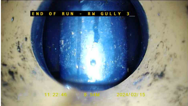
aff5abb1-d8bc-42d0-b147-c52168b645ee.jpg, 00:01:27, 8.54 m Finish node, gully, reference: Branch A, RWG3
