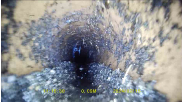
4ebcb5db-0fa7-472b-9e97-0df6afe2e321.jpg, 00:00:11, 0.01 m Settled deposits, fine, 20% cross-sectional area loss, start
