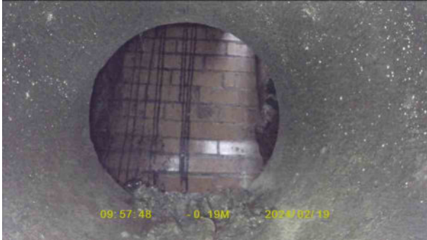
a193fc46-fa23-471b-ba4e-6ba2f7f41d1e.jpg, 00:00:14, 0.19 m Settled deposits, fine, 15% cross-sectional area loss
