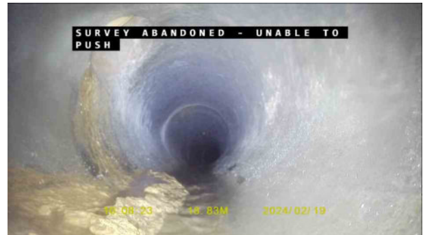
de9b4cd7-f0d2-432a-b32e-be68fcb09be2.jpg, 00:07:00, 18.83 m Survey abandoned, Camera unable to push further
