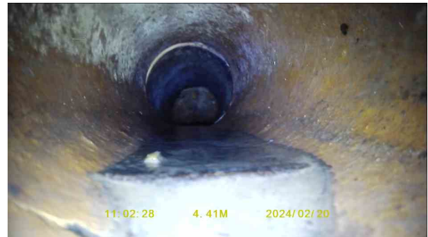
46a8db89-2395-4346-b1ab-494535b5cd78.jpg, 00:01:02, 4.41 m Attached deposits, encrustation from 5 o'clock to 7 o'clock,
