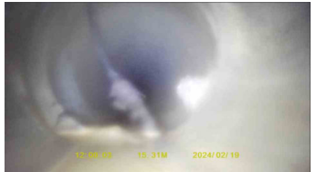
5bc5e9c3-7372-459e-bec9-e99023f639ba.jpg, 00:01:44, 15.51 m Joint displaced, large
