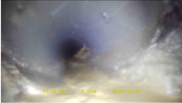
7a5d2fc7-f41c-4101-9c53-568f3bec3a03.jpg, 00:00:14, 0.96 m Attached deposits, encrustation at joint from 2 o'clock to 7 o'clock, 20% cross-sectional area loss, start
