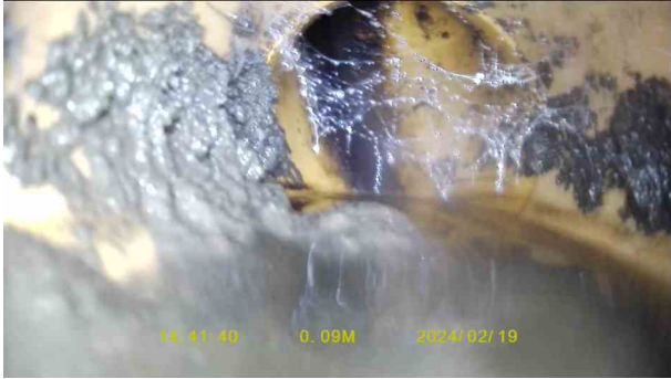
f07e7265-1a78-4885-83d7-e3071f993674.jpg, 00:00:10, 0.09 m Settled deposits, fine, 15% cross-sectional area loss
