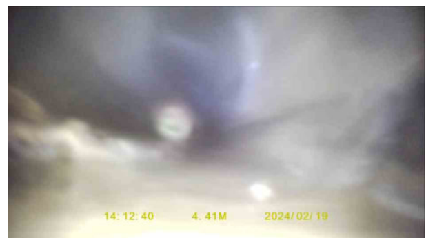
2cc2f0bb-4106-4f9a-aa5e-a43e4c66eafe.jpg, 00:00:56, 4.41 m Roots, tap at joint
