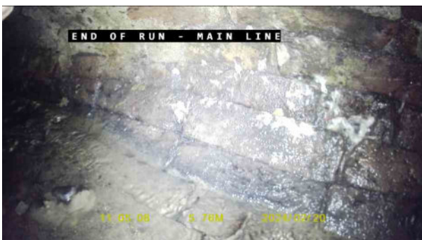
e878b872-6e34-410d-afb7-adb481f5e729.jpg, 00:01:32, 5.76 m Finish node, manhole, reference: Main line
