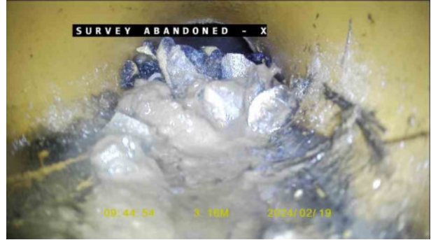
0f000214-7f3c-4309-82b6-efbfe00a12e8.jpg, 00:00:49, 3.16 m Survey abandoned, Camera unable to pass debris
