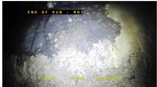
5c05eb00-58fe-4748-9f19-052cce5bfb2e.jpg, 00:02:10, 10.58 m Finish node, manhole, reference: MH2
