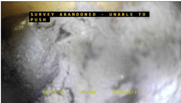
b3d517be-2c67-4ef1-a381-ccbc479d77ed.jpg, 00:00:58, 0.19 m Survey abandoned, Camera unable to pass debris
