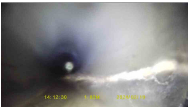
5769829f-e1f7-44b6-84d6-26706f8fbbf2.jpg, 00:00:46, 1.82 m Roots, tap at joint
