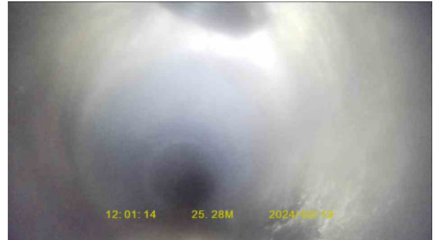
5c7aa283-64f9-4da0-b400-cf3cc3160b30.jpg, 00:02:54, 25.28 m Junction at 1 o'clock, 150mm dia
