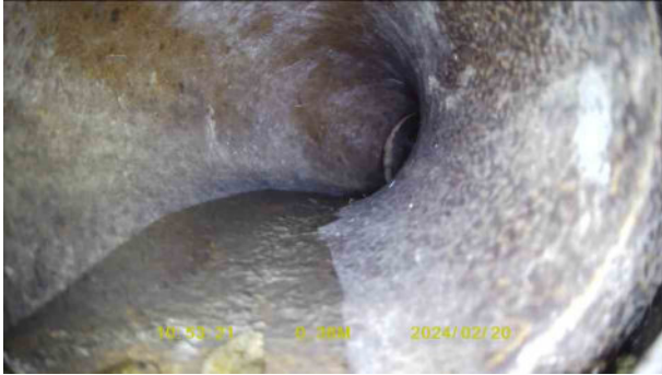
94c4cd49-8989-4d64-ba70-694f6b00c783.jpg, 00:00:15, 0.38 m Joint displaced, medium
