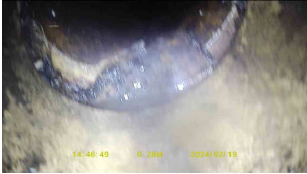
19414010-d444-4786-ba73-fbb897affb06.jpg, 00:00:18, 0.28 m Joint displaced, large
