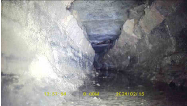
fe6ca740-4cf9-47e2-9136-ef9903ed7e3e.jpg, 00:00:09, 0.01 m Hole in drain or sewer from 10 o'clock to 2 o'clock, start
