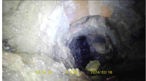
548a9801-4d4e-4b9c-8021-e88d28ad1322.jpg, 00:00:18, 0.57 m Settled deposits, fine, 20% cross-sectional area loss, start
