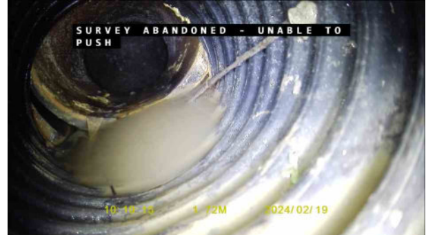
46a9c229-a384-4b90-8825-e392ff907ccf.jpg, 00:01:00, 1.72 m Joint displaced, large
