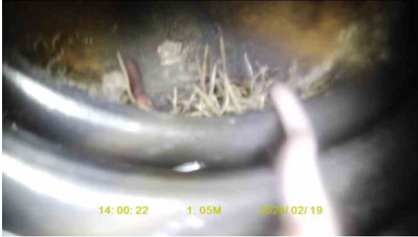
75738fd2-057a-42e3-8af6-84ea17b29526.jpg, 00:00:21, 1.05 m Roots, fine at joint
