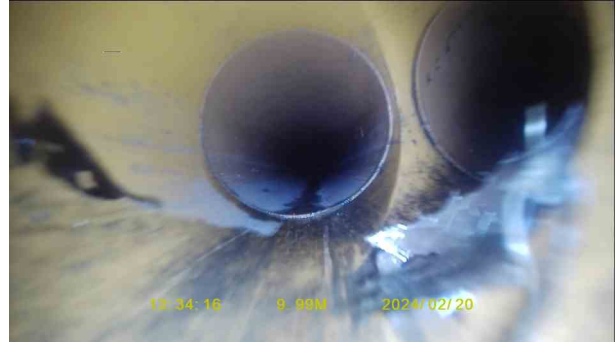
f28f0d2e-5a81-457a-95b7-6385d09598fa.jpg, 00:01:41, 9.99 m Junction at 3 o'clock, 100mm dia
