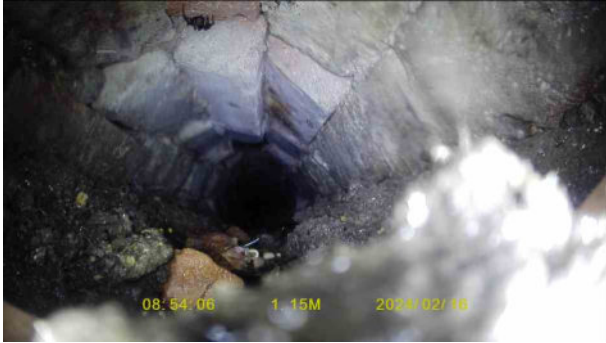
84b0b716-2f8d-4276-9b3f-552035c7ef7e.jpg, 00:00:19, 1.15 m Settled deposits, coarse, 20% cross-sectional area loss, start
