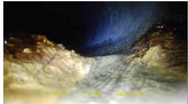
73255367-82f0-46a0-ae9f-d90a988d73ae.jpg, 00:02:14, 13.72 m Attached deposits, encrustation from 3 o'clock to 5 o'clock,
