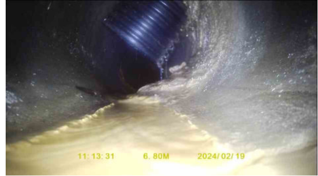
9fe7f2ed-5c9a-4730-af14-163464b89487.jpg, 00:01:37, 6.80 m Connection defective, connecting pipe is intruding at 1 o'clock,
