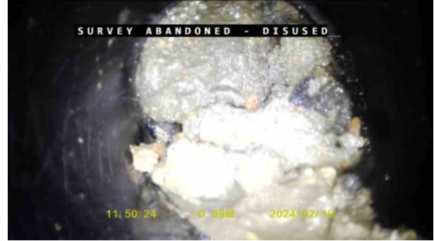
77bd05ec-a575-4cef-8f06-9d9bc9e019ed.jpg, 00:00:12, 0.09 m Survey abandoned, Disused
