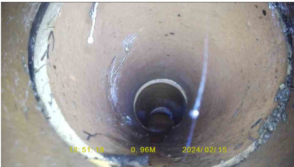
7b959420-30df-46fe-8b1c-021aa6c8dd4c.jpg, 00:00:28, 0.96 m Joint displaced, medium
