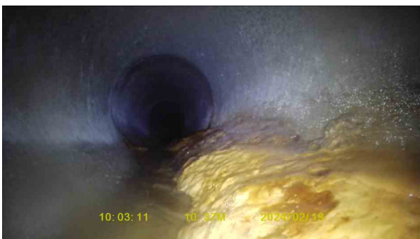
4af5cef2-5db1-4131-aa13-0ebe6428aa7f.jpg, 00:02:43, 10.00 m Attached deposits, encrustation from 3 o'clock to 6 o'clock,
