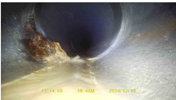
974cc9ab-f178-4677-8b46-f403d2fa1616.jpg, 00:02:11, 10.48 m Attached deposits, encrustation at joint from 7 o'clock to 9
