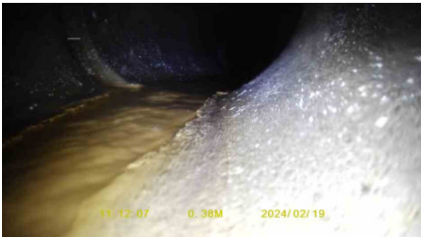
43fb38b2-6110-4a95-8fd4-09d5dc22a300.jpg, 00:00:13, 0.38 m Joint displaced, medium
