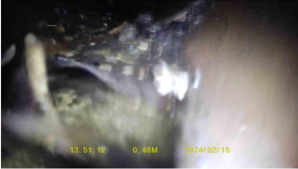
20c95e4e-6e9c-4eee-b96d-9d31401beb11.jpg, 00:00:22, 0.48 m Settled deposits, fine, 25% cross-sectional area loss, start
