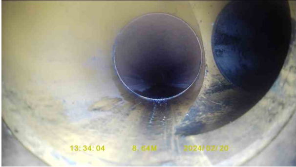
1cff4279-29bc-41d9-a284-c0b1df4fa83c.jpg, 00:01:28, 8.64 m Junction at 3 o'clock, 100mm dia
