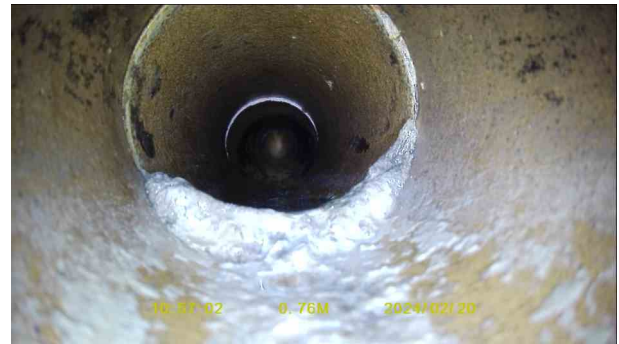
c49eab87-a58d-4fd3-9800-c705466255a4.jpg, 00:00:26, 0.76 m Attached deposits, encrustation at joint from 4 o'clock to 7
