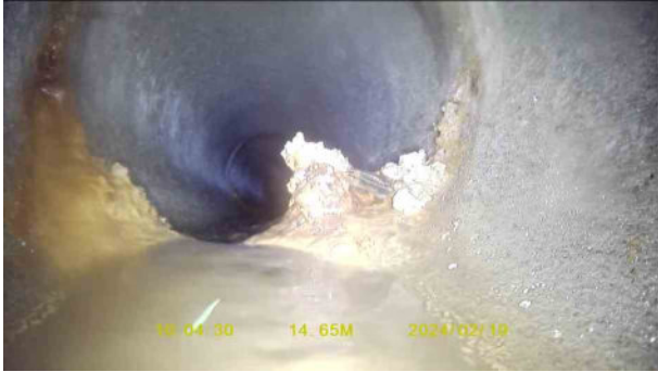
9b1df465-ba5a-4281-bed4-713f3c375753.jpg, 00:04:53, 14.65 m Attached deposits, encrustation at joint from 3 o'clock to 7
