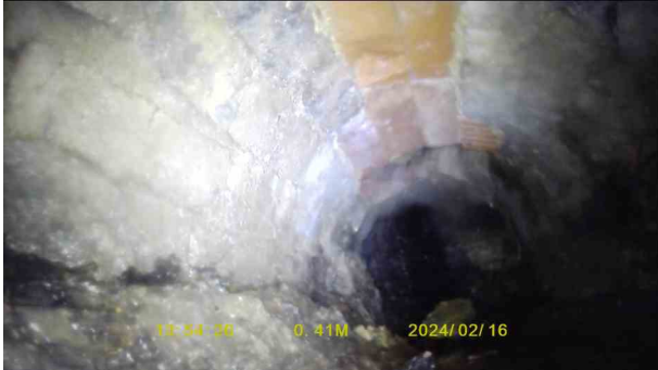
4ef6300e-2f9d-4306-95ef-b6cd0994d147.jpg, 00:00:14, 0.41 m Broken pipe from 8 o'clock to 9 o'clock, start
