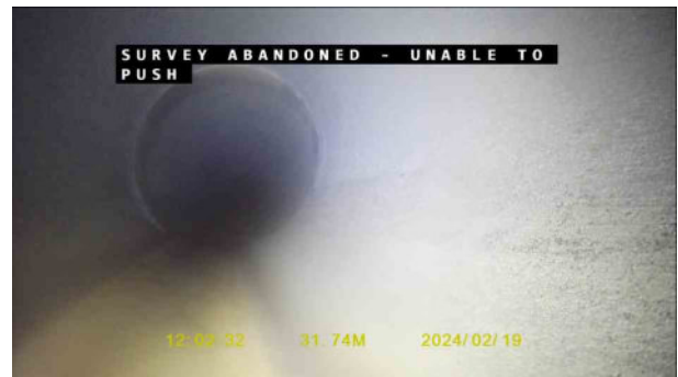
fad08eb9-8ce5-4b49-812a-45c4178156dd.jpg, 00:03:44, 31.74 m Survey abandoned, Camera unable to push further
