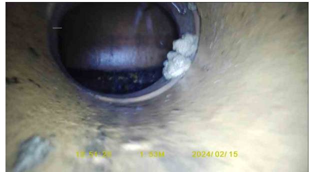
f1f2450b-46f3-4ac6-8aa2-235a2dc617f9.jpg, 00:00:34, 1.53 m Attached deposits, encrustation at joint from 3 o'clock to 4 o'clock, 15% cross-sectional area loss
