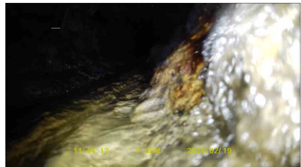
ed780d85-16dd-4e26-8e1c-0f15d63ba222.jpg, 00:02:16, 7.05 m Attached deposits, encrustation from 3 o'clock to 7 o'clock,
