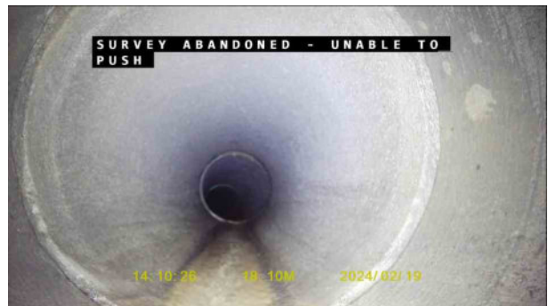
bd9add86-3620-47fd-a734-39fc3966ba3d.jpg, 00:02:29, 18.10 m Survey abandoned, Camera unable to push further
