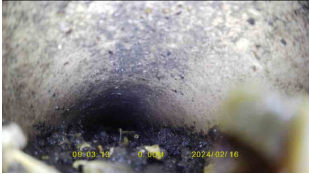
ba401d94-9d63-4eab-954e-07c8f4bf1f0e.jpg, 00:00:10, 0.01 m Settled deposits, fine, 60% cross-sectional area loss, start
