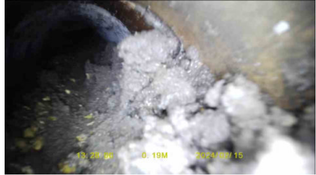
1c44eae0-37b6-4678-8aee-5aa4b04f4063.jpg, 00:00:20, 0.19 m Settled deposits, fine, 50% cross-sectional area loss, start
