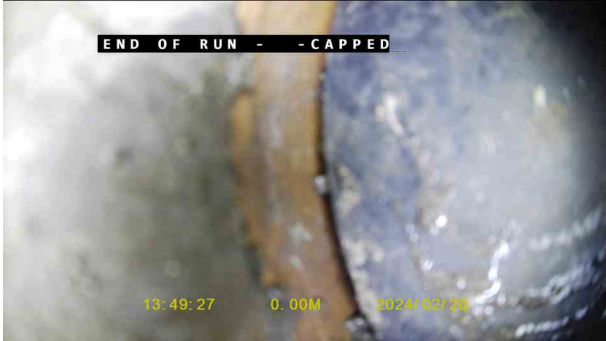
fc91452-5e55-4616-9fb5-a1479d9cbaa1.jpg, 00:00:39, 0.01 m Finish node, manhole, reference: Capped
