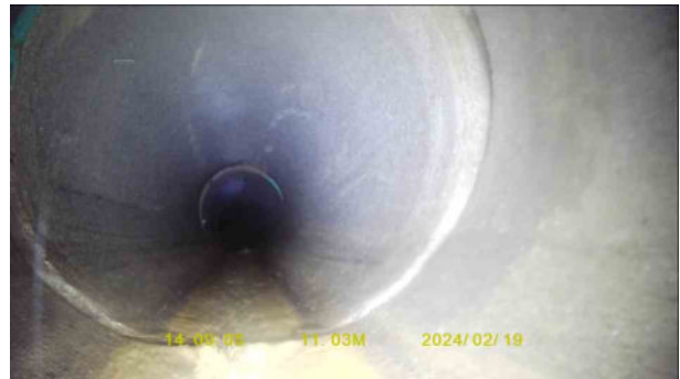
c0b29321-b805-4a0e-ad8a-f4155bced4b7.jpg, 00:01:41, 11.03 m Joint displaced, medium
