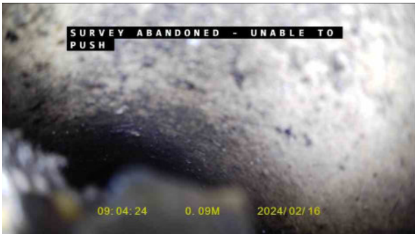
73afe08c-7a2a-4d40-8ce3-037b55db0272.jpg, 00:00:41, 0.19 m Survey abandoned, Camera unable to pass debris
