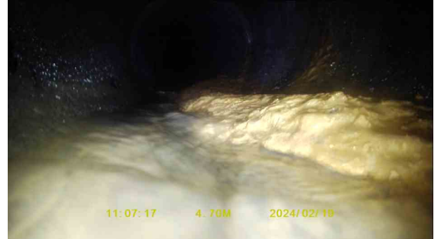
ac3e9b83-6581-407c-a00c-a1c81769c22a.jpg, 00:01:01, 4.70 m Attached deposits, encrustation from 3 o'clock to 5 o'clock,
