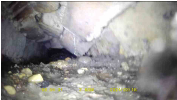
e31a2e52-a6f1-4f0a-b689-c60b44c4b2d1.jpg, 00:00:44, 2.69 m Settled deposits, coarse, 40% cross-sectional area loss,
