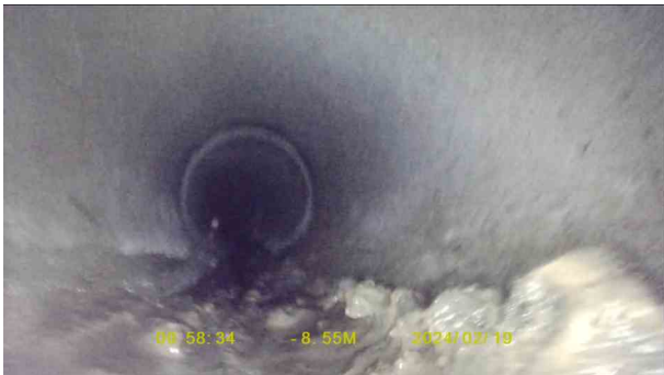
1cdcae68-ac06-4b81-8169-bb18b55dd423.jpg, 00:01:00, 8.55 m Settled deposits, fine, 20% cross-sectional area loss, start
