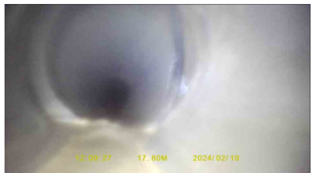
077590d8-4c9b-4e1f-9992-55e9dadfdb62.jpg, 00:02:08, 17.89 m Joint displaced, large
