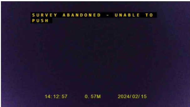
7e3b7bc0-30c8-42e8-9e52-30451373290b.jpg, 00:00:42, 0.57 m Survey abandoned, Loss of vision due to debris
