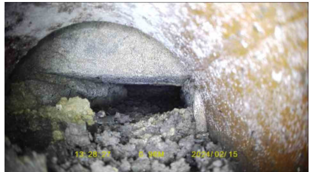
f0cc2763-8207-4804-a4ab-e36e04128bba.jpg, 00:00:41, 0.96 m Survey abandoned, Camera unable to push further
