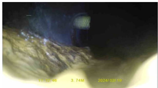
25429ab5-a586-4df5-9b40-2c0439df4630.jpg, 00:00:53, 3.74 m Connection defective, connecting pipe is intruding at 10
