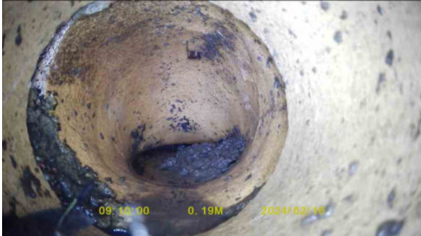
8f0bf5e6-2d78-4aa6-8b3c-8a2c8bccca296.jpg, 00:00:20, 0.19 m Joint displaced, medium
