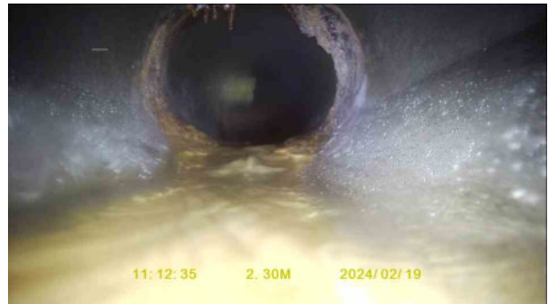
32e4f982-7d43-48bf-8c44-f932a7952cc4.jpg, 00:00:41, 2.30 m Attached deposits, encrustation at joint from 12 o'clock to 12 o'clock, 15% cross-sectional area loss
