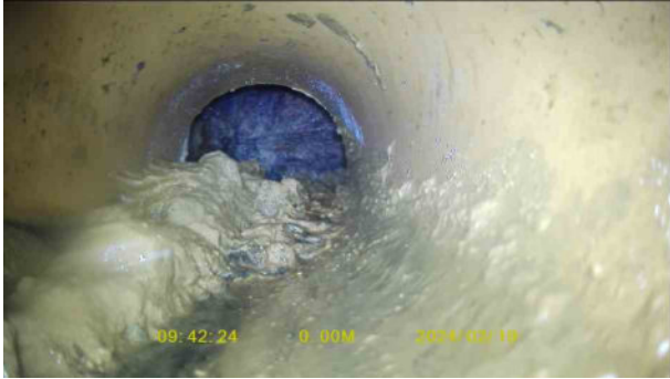
bd3cb6e8-d3e1-4268-9cfc-2e375bdc3a05.jpg, 00:00:11, 0.01 m Settled deposits, fine, 30% cross-sectional area loss, start
