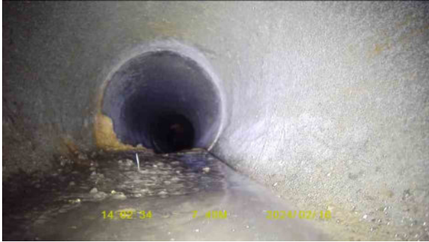
3d1525e2-dcc1-4be8-9519-7761d187d133.jpg, 00:01:04, 7.49 m Settled deposits, fine, 20% cross-sectional area loss, start
