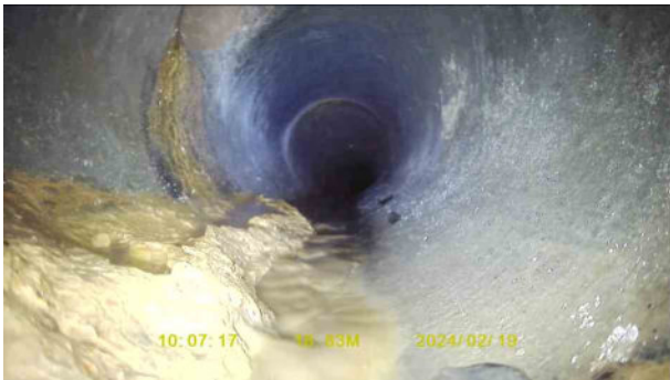
5fc6656d-dacf-4208-bb80-f0a318aef99e.jpg, 00:06:04, 18.83 m Junction at 11 o'clock, 100mm dia
