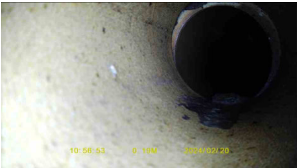
205e2d51-6137-455f-aa65-6f6f489f32b0.jpg, 00:00:18, 0.28 m Joint displaced, medium
