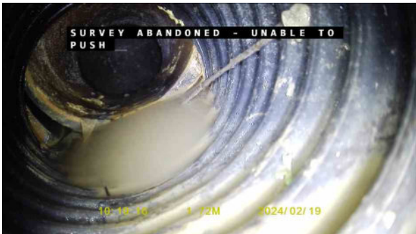
a12f9621-363e-4716-a179-4259851e7146.jpg, 00:01:00, 1.72 m Open joint, large
