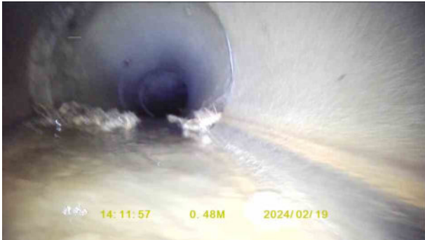
9ef8f719-6f34-4061-9c71-530c3ecf69fb.jpg, 00:00:12, 0.48 m Joint displaced, large
