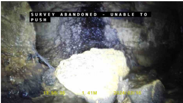
0231ad88-5588-41bb-b1e0-f9aa52024e8c.jpg, 00:01:04, 1.41 m Settled deposits, coarse, 30% cross-sectional area loss
