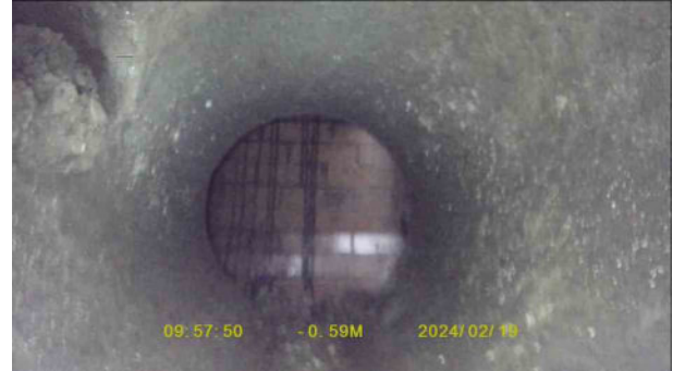
7d35edb2-a981-4e3e-9490-ae5dee594a66.jpg, 00:00:16, 0.59 m Junction, blocked at 10 o'clock, 150mm dia
