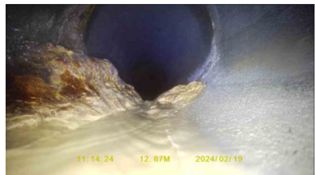
22f12925-390f-4c45-80db-538b3d662c09.jpg, 00:02:31, 12.87 m Attached deposits, encrustation at joint from 4 o'clock to 11
