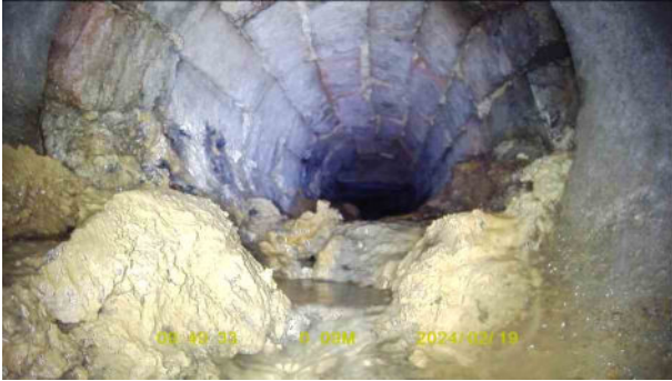
2749778e-e127-4fee-85d2-547ac9196837.jpg, 00:00:14, 0.09 m Settled deposits, coarse, 40% cross-sectional area loss, start
