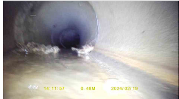
66386fb9-964f-40e2-b990-b4504dcca0eb.jpg, 00:00:12, 0.48 m Attached deposits, encrustation at joint from 5 o'clock to 8
