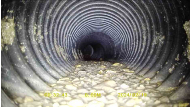
a2dc3797-f61a-4ba7-bb9a-1e1d3a959971.jpg, 00:00:11, 0.01 m Settled deposits, fine, 20% cross-sectional area loss, start
