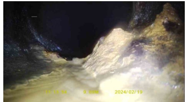
25845356-a660-487b-aea4-d6a70e377d5f.jpg, 00:02:00, 9.09 m Attached deposits, encrustation at joint from 4 o'clock to 8
