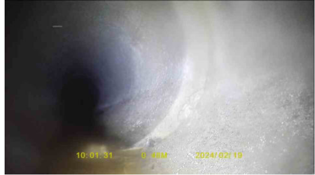
577c0377-0c71-499c-9544-72f3aa53bc83.jpg, 00:01:03, 0.38 m Joint displaced, medium
