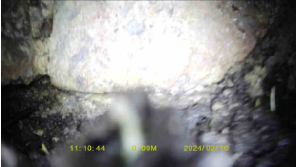
f02a77e9-e2f1-4c09-8064-3d1f006b46ec.jpg, 00:00:26, 0.09 m Settled deposits, fine, 30% cross-sectional area loss
