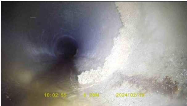
40adf8c3-9121-4654-9bc3-ba28ca5e23bb.jpg, 00:02:26, 8.28 m Attached deposits, encrustation at joint from 12 o'clock to 5
