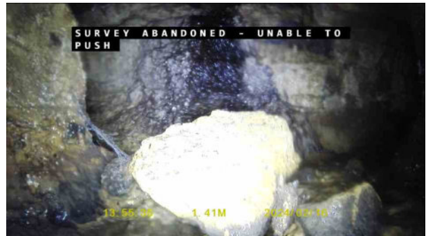
e442f1d8-f945-4c7a-9174-83f5532d3724.jpg, 00:01:04, 1.41 m Survey abandoned, Camera unable to push further
