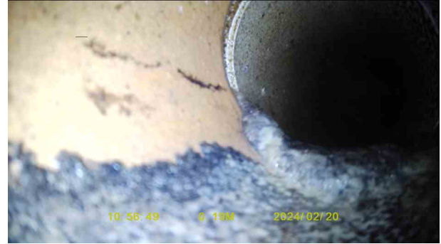
4bff65e0-e500-4552-8682-5a6f3d023944.jpg, 00:00:14, 0.19 m Attached deposits, encrustation at joint from 4 o'clock to 8
