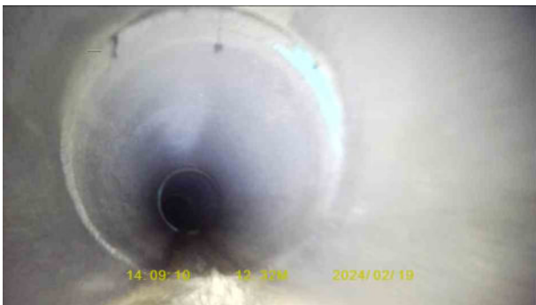
e3ef380b-964e-4a72-a3f0-f538712dbf1e.jpg, 00:01:47, 12.32 m Joint displaced, medium
