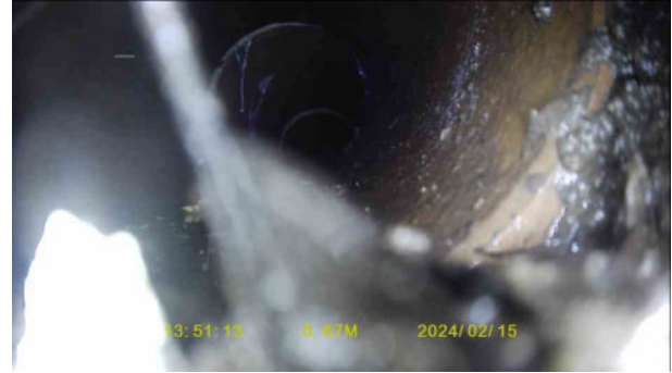
afcd81bb-6da3-4ec1-b5c4-cda859859e55.jpg, 00:00:23, 0.67 m Joint displaced, large
