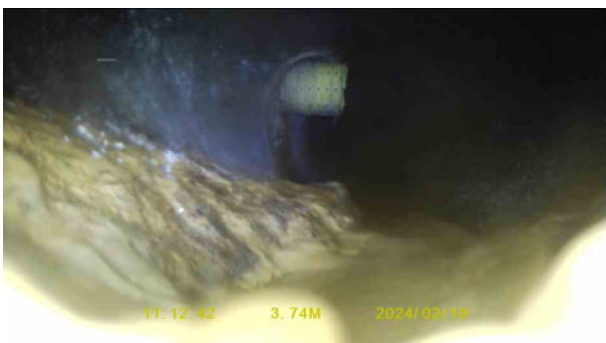
e94015b3-ed59-45f9-848b-a6e22f99c630.jpg, 00:00:48, 3.74 m Attached deposits, encrustation from 6 o'clock to 9 o'clock,
