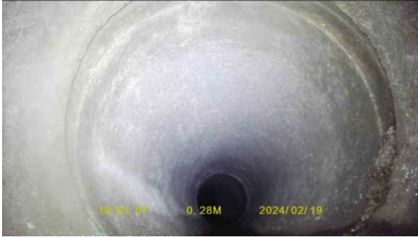
665fee94-ec28-4250-ae46-7b492f39d699.jpg, 00:00:39, 0.28 m Joint displaced, medium
