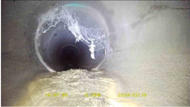
c90c49cb-90c8-4c29-b9e6-25c9edb953bc.jpg, 00:00:15, 0.28 m Settled deposits, fine, 20% cross-sectional area loss
