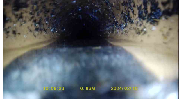
9139b476-f04d-427c-b933-e8b7d94a1fc7.jpg, 00:00:24, 0.86 m Settled deposits, fine, 20% cross-sectional area loss, start
