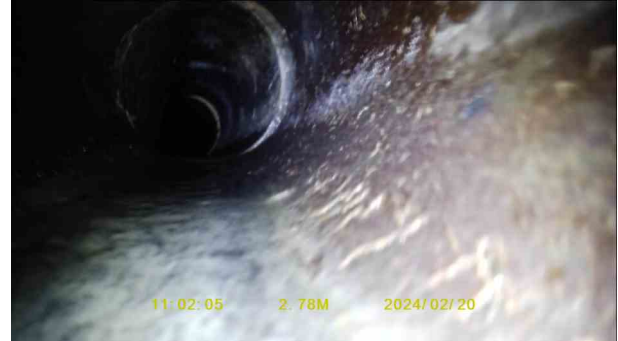
f655621c-2490-4b57-b90c-2478f909dfd8.jpg, 00:00:39, 2.78 m Joint displaced, medium
