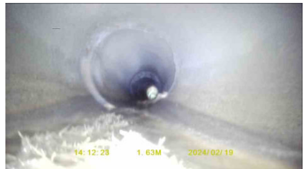
979dab86-6af4-43fd-83df-ea5f15483789.jpg, 00:00:39, 1.63 m Joint displaced, large
