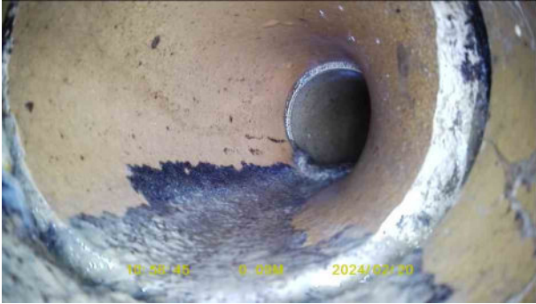
7076801a-6240-41d9-a416-603246e932b2.jpg, 00:00:10, 0.09 m Joint displaced, medium
