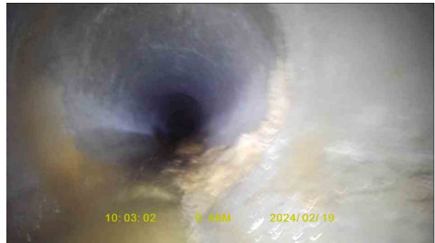
ec57c0d9-4e86-40a5-b827-5f5e43b77d41.jpg, 00:02:34, 9.68 m Attached deposits, encrustation at joint from 3 o'clock to 8
