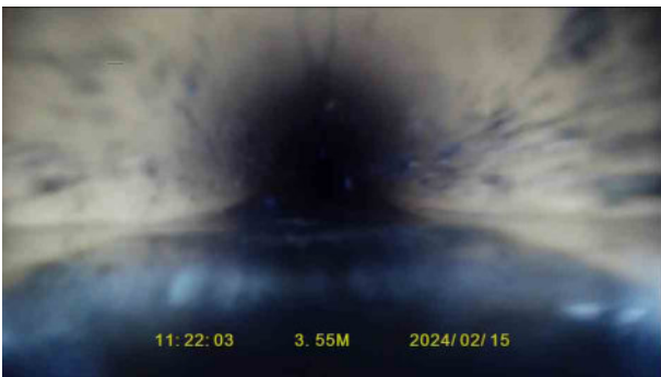
ea51794f-0e49-406f-a021-baaee9d72fa0.jpg, 00:00:47, 3.55 m Settled deposits, fine, 20% cross-sectional area loss, start
