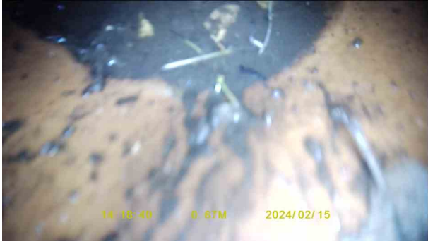
ccde89bb-de1f-44ef-bd98-8822d6aa2ec0.jpg, 00:00:28, 0.67 m Settled deposits, fine, 25% cross-sectional area loss, start
