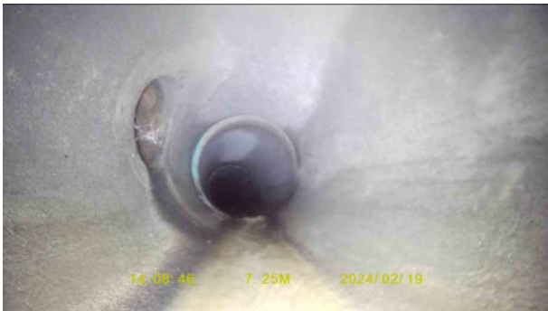
ed25be0b-d9fb-40a3-b387-61b8707a9e33.jpg, 00:01:22, 7.25 m Junction at 9 o'clock, 150mm dia
