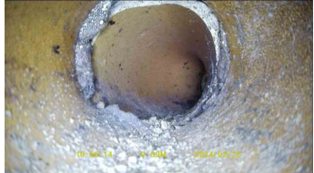
e02efbb9-b02d-404c-88dc-d7230a88ceff.jpg, 00:00:13, 0.09 m Broken pipe at joint from 9 o'clock to 4 o'clock
