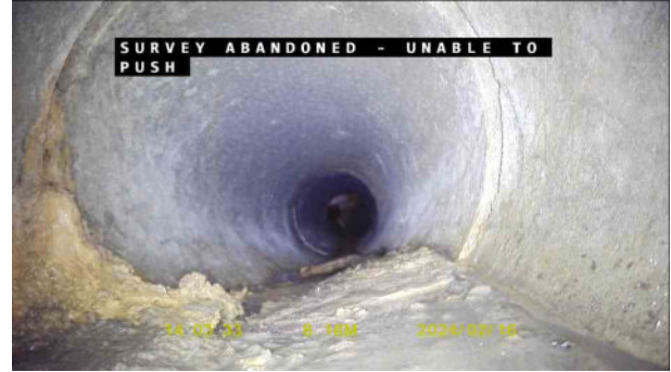
a0e355cb-3626-4767-b647-5fba654fe9cd.jpg, 00:01:59, 8.16 m Survey abandoned, Camera unable to pass debris
