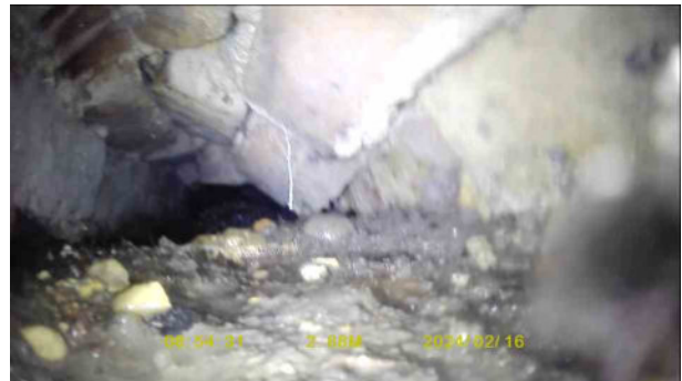
7935c141-1592-43c0-a41b-1905a285488e.jpg, 00:00:44, 2.69 m Displaced bricks, single brick False from 9 o'clock to 3 o'clock,
