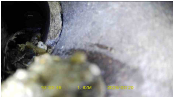
d2831d65-8e38-403f-8a5f-c8cc4d858d74.jpg, 00:00:42, 1.82 m Joint displaced, medium
