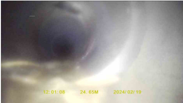
48778814-9246-4c73-ba73-c912ead5b075.jpg, 00:02:49, 24.65 m Joint displaced, large
