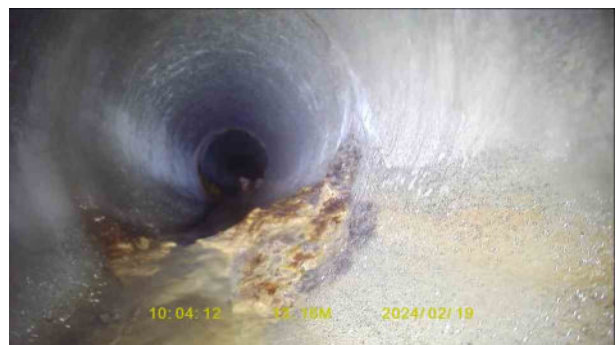
f43cf5ae-dbc6-46d7-a8e2-2457b71d9616.jpg, 00:03:44, 13.16 m Attached deposits, encrustation at joint from 3 o'clock to 8
