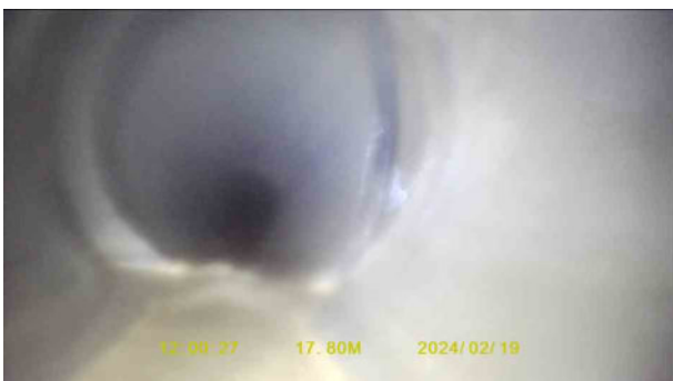
6aaf9e92-ed2e-4459-af05-5463ec3b53e4.jpg, 00:02:08, 17.89 m Roots, tap at joint
