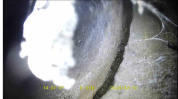
ef996390-ddfa-4960-9671-61ea9d940e87.jpg, 00:00:24, 0.67 m Joint displaced, medium
