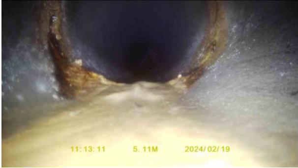
d7657106-80da-4f98-885f-3660c731a98d.jpg, 00:01:17, 5.11 m Attached deposits, encrustation at joint from 12 o'clock to 12
