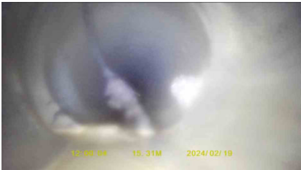
cfd37089-f5b5-48ce-ac96-437949ebdf9e.jpg, 00:01:44, 15.31 m Roots, tap at joint
