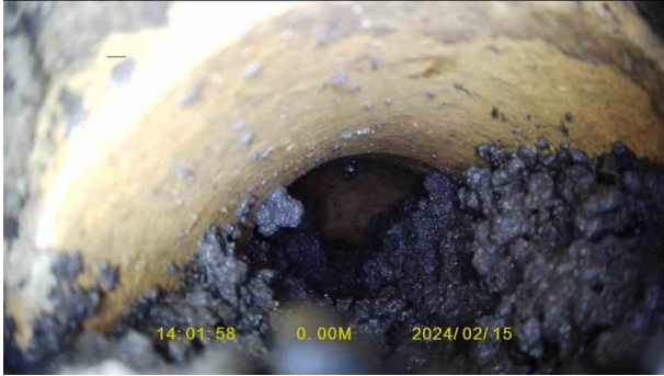
7ba87c9a-6b39-42d4-ae10-ec3c1a5078b6.jpg, 00:00:19, 0.01 m Settled deposits, fine, 30% cross-sectional area loss
