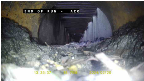
863abe23-34c2-4e95-8c46-44d1baf7e004.jpg, 00:02:46, 18.75 m Settled deposits, fine, 45% cross-sectional area loss, Aco
