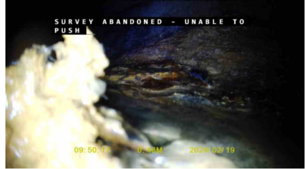
d284b3ad-28d3-422e-9f95-585843d0d021.jpg, 00:00:39, 0.48 m Survey abandoned, Camera unable to pass debris
