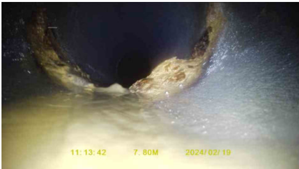
2e4e80b4-c8d3-4cd7-ae00-f610bb2f986c.jpg, 00:01:49, 7.80 m Attached deposits, encrustation at joint from 12 o'clock to 12
