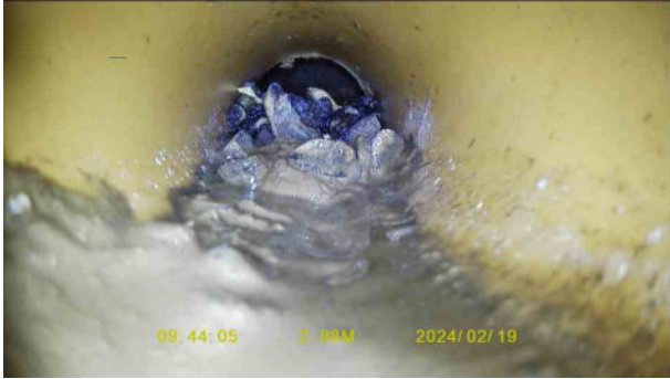
f4d6a904-8467-4fc3-94f9-5545c6fd43c2.jpg, 00:00:36, 2.88 m Settled deposits, coarse, 70% cross-sectional area loss
