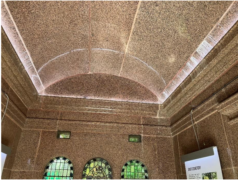
Photograph 12: Strathcona vault interior – mortar leaching is visible
