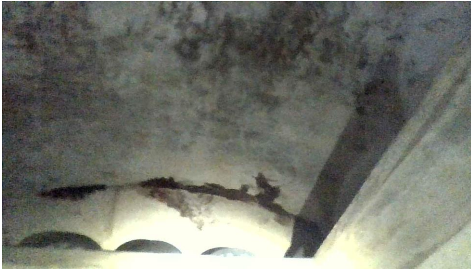
Photograph 5: Outer Circle Vault 13 (Brett) – typical dampness at vault intrados
