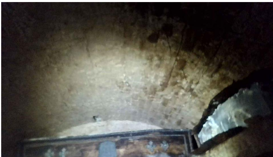
Photograph 7: Egyptian Avenue – typical view of brick vault intrados showing some dampness and limited fine root penetration.
