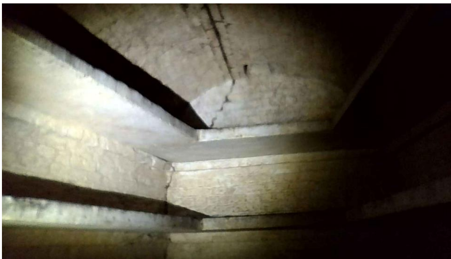
Photograph 4: Inner Circle Vault 1: Typical example of longitudinal cracking at the vault intrados and more isolated example of cracking to the rear wall.
