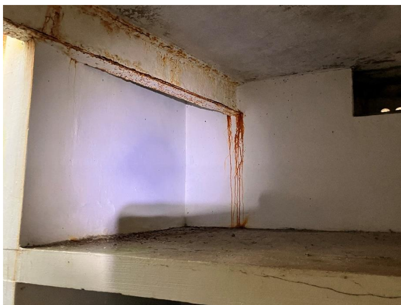
Photograph 16: Otway Vault – example of water ingress at steel beam bearing
