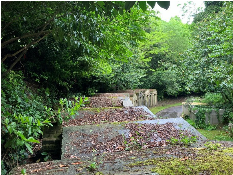
Photograph 11: General view of roof slabs at the north end of the row.
