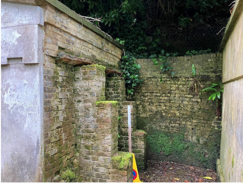
Photograph 10: External buttressing to the Hawes vault with saturated brickwork to the visible retaining wall on the right.
