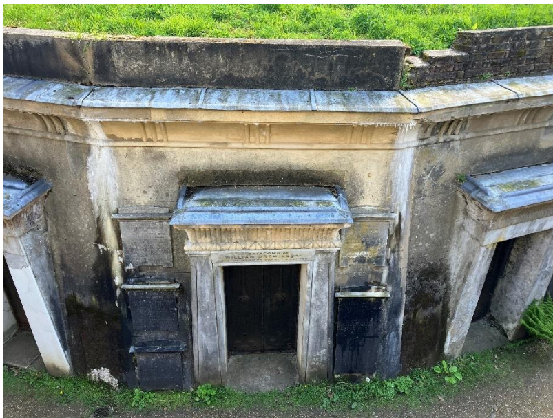
Photograph 6: Inner Circle – example of mortar washout at parapet level and dampness at low level due to drainage issues.
