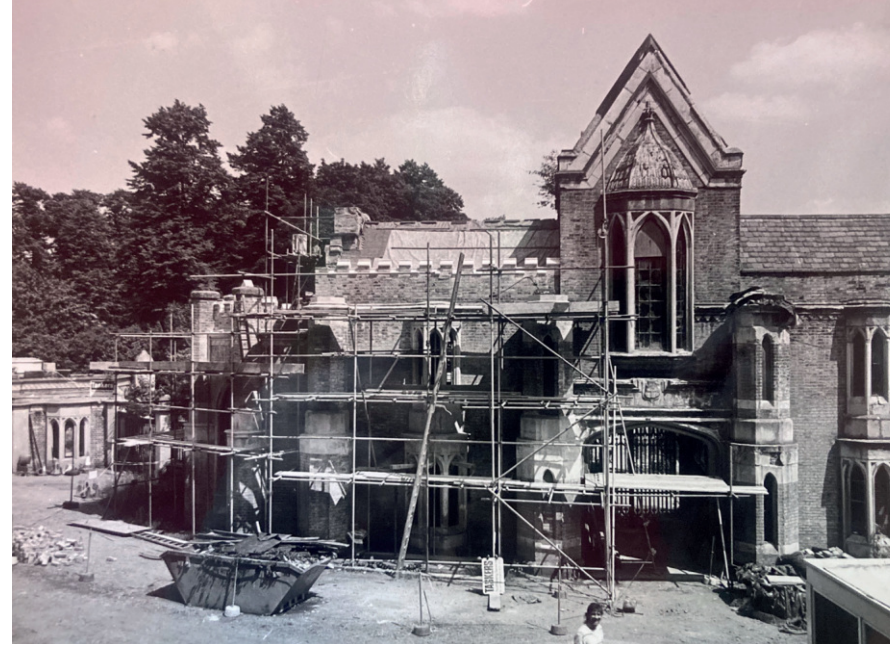
Figure 7.21 Photograph of the Chapel during repair works. Undated but likely taken by Gay in the 1980s (source: FoHCT Archives)
