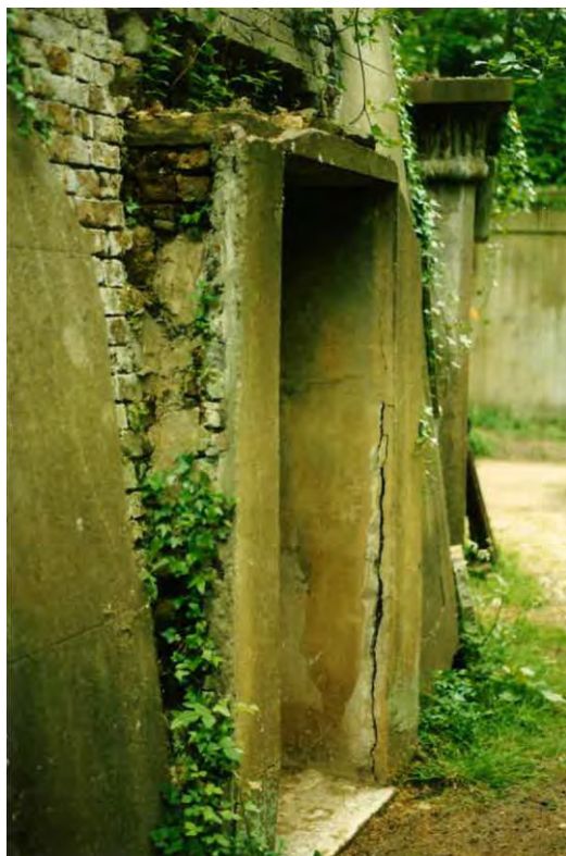
Figure 6: Decayed state of Vault 13 doorway prior to conservation
