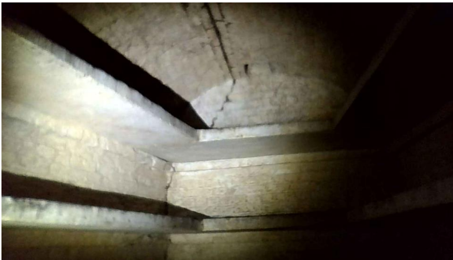
Photograph 4: Inner Circle Vault 1: Typical example of longitudinal cracking at the vault intrados and more isolated example of cracking to the rear wall.
