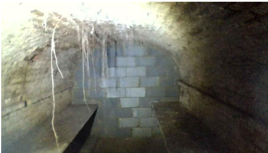
Photograph 2: Unnamed vault at eastern end – root penetration and probable cracking to the vault intrados.
