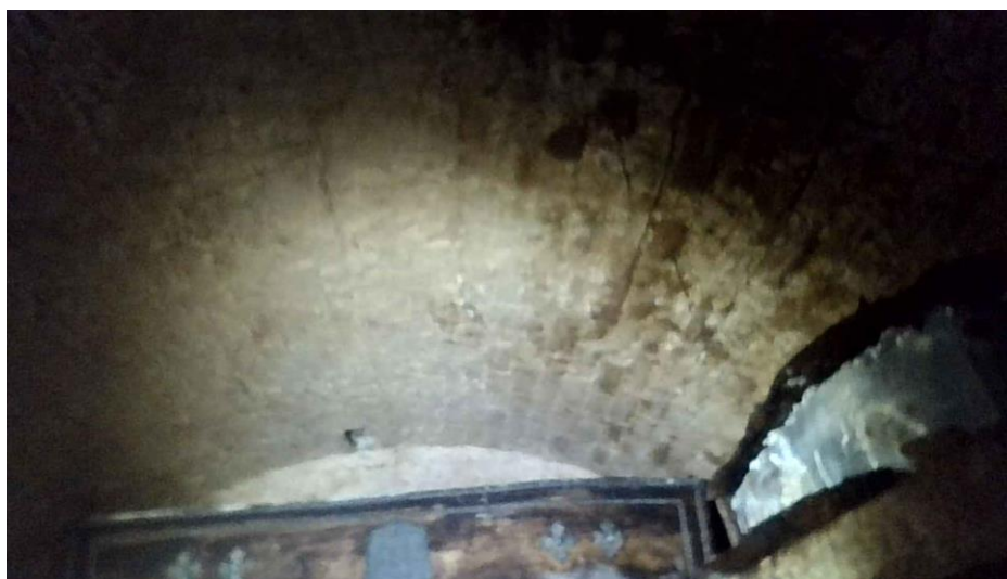
Photograph 7: Egyptian Avenue – typical view of brick vault intrados showing some dampness and limited fine root penetration.
