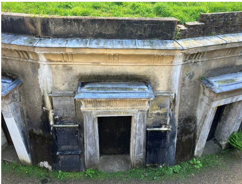
Photograph 6: Inner Circle – example of mortar washout at parapet level and dampness at low level due to drainage issues.
