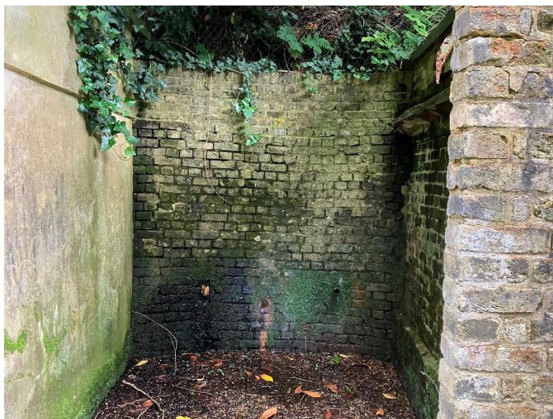
Photograph 11: Water draining out through existing weep holes and brickwork joints and ponding on the ground under.
