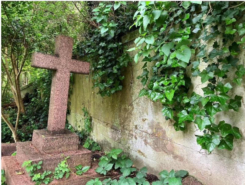
Photograph 3: Failing retaining wall at western end of the Terrace Catacombs.
