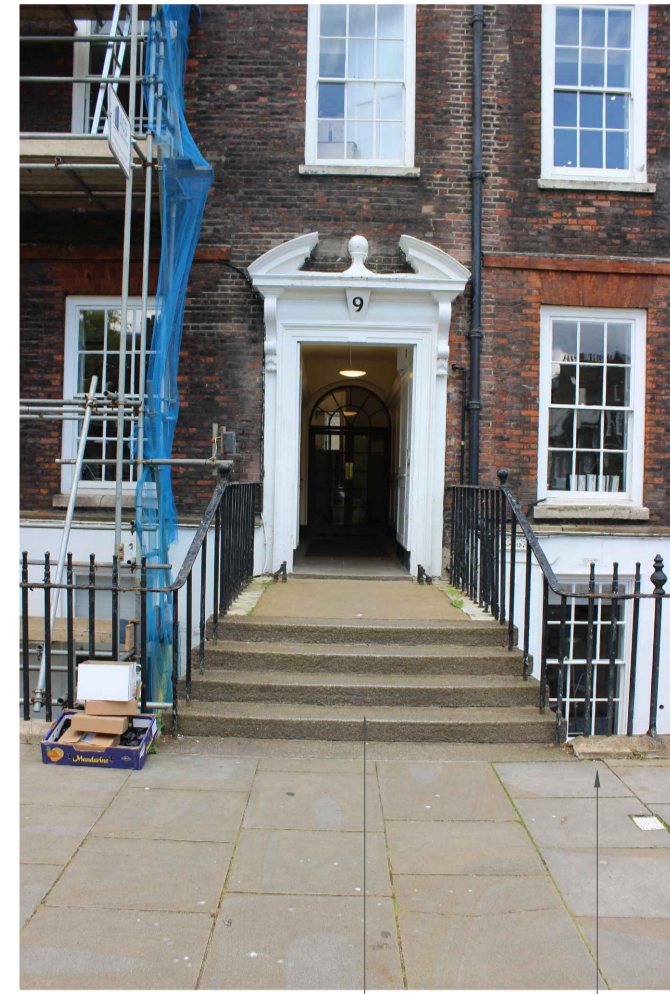
Open joints need repointing (NHL 5.0)
