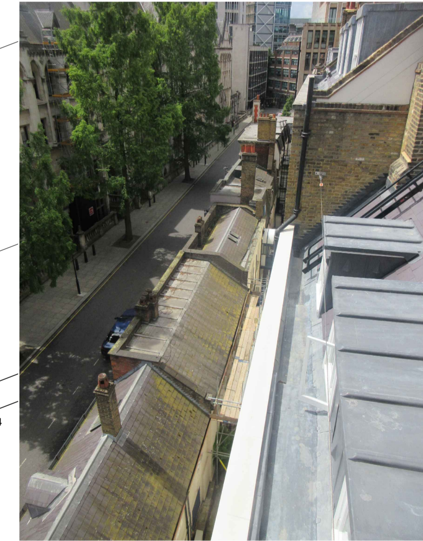
New stainless steel harness fixing point.
