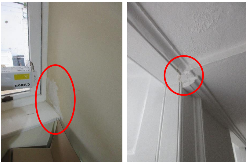
Above left: Damp to window reveal under entrance bridge. Room 9NS/B11. Above right: Small area of moisture staining above WB06 in Room 9NS/B6.
