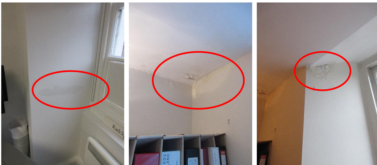
Above left: Damp patch to north side of WB02 in Room 11NS/B5.
