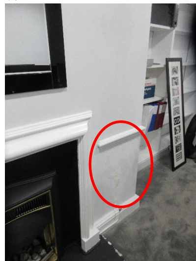
Above right: Damp patch to the east of the fireplace in Room 11NS/B10.
