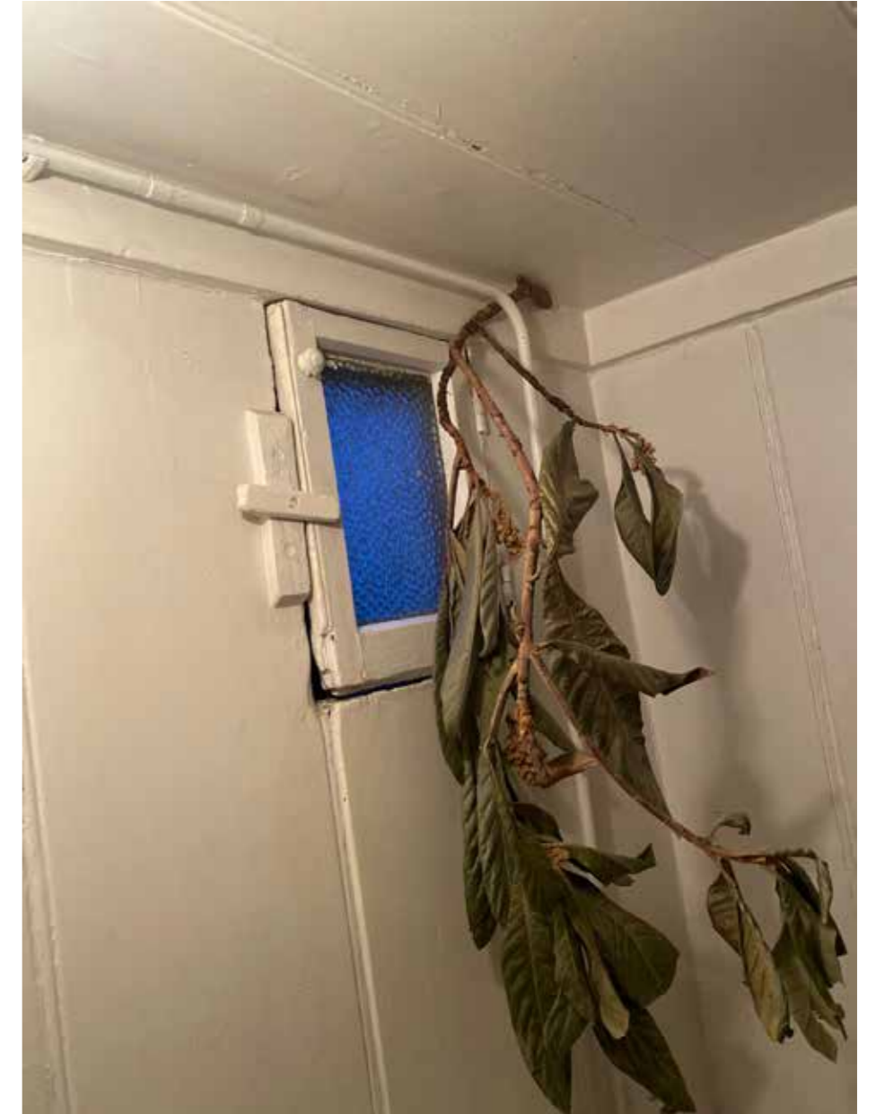
Figure 3.16 Photograph of the interior of the WC, showing the butt and bead panelling and small hatch window.
