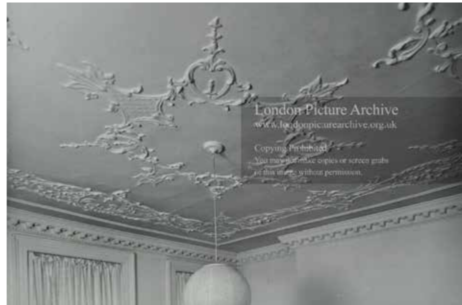
Figure 3.12 Original cornicing and ceiling rose shown in the neighbouring No.26 Charlotte Street, 1974. Source: London Picture Archive.
