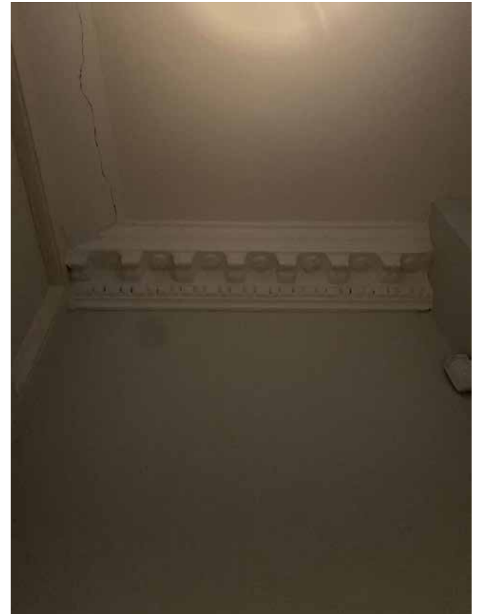
Figure 3.13 Remnants of original cornicing in the first floor hallway of 28 Charlotte Street.
