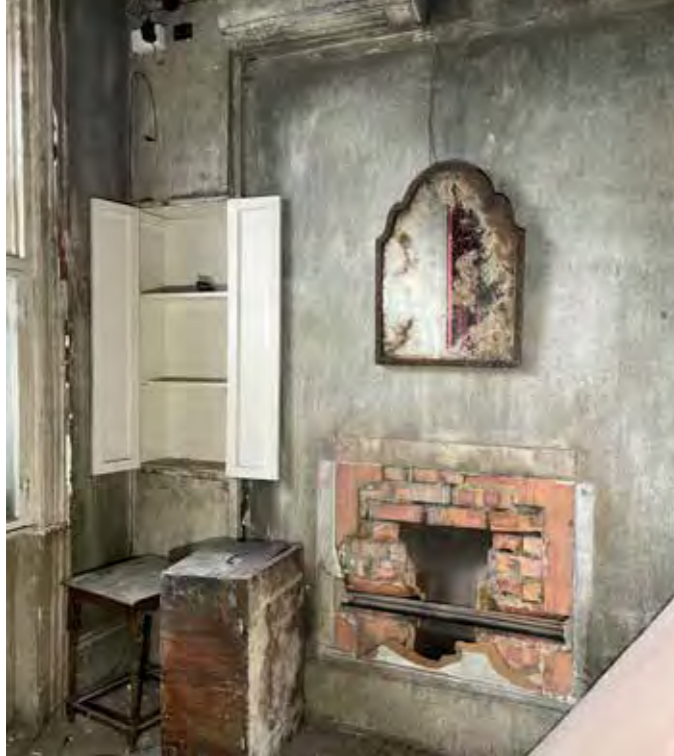
Infilled fireplace with pre-war common bricks - evidence of c1930s phase. Cupboard with modern joinery
