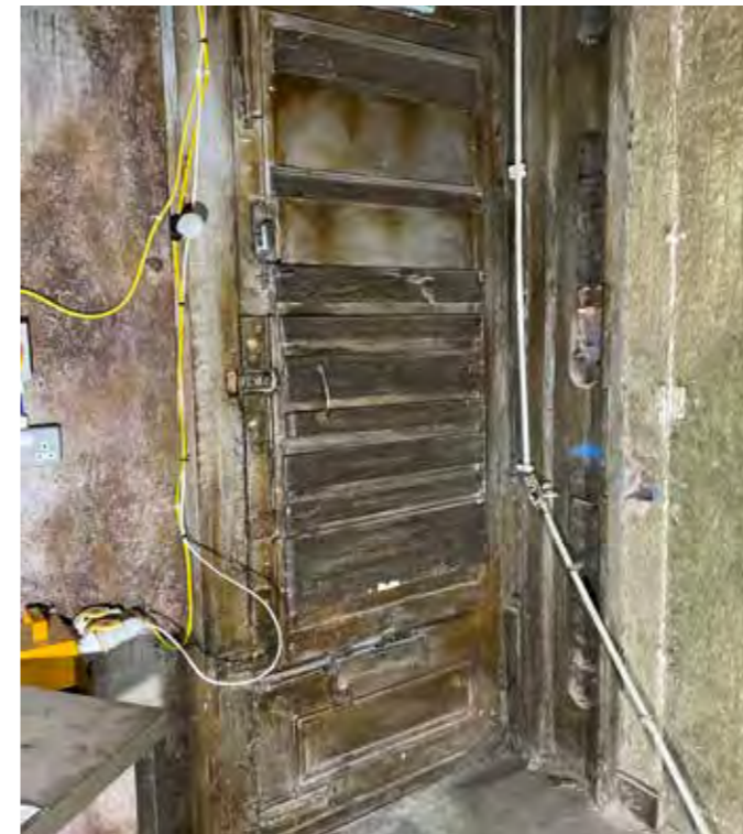
Door to shopfront, some early fabric, phases of ironmongery alteration.
