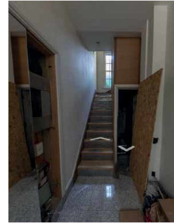
Ground floor of no. 12. Fitted mirror and stair treads, panels, and risers excluded from listing
