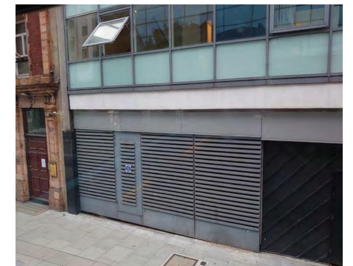
Existing UKPN Substation on High Holborn
