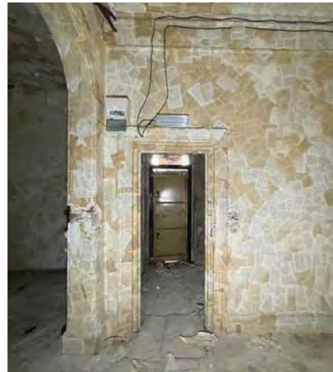
Cornice, Skirting & architrave all of early phases Arch with c1860s details joining front and back rooms.
