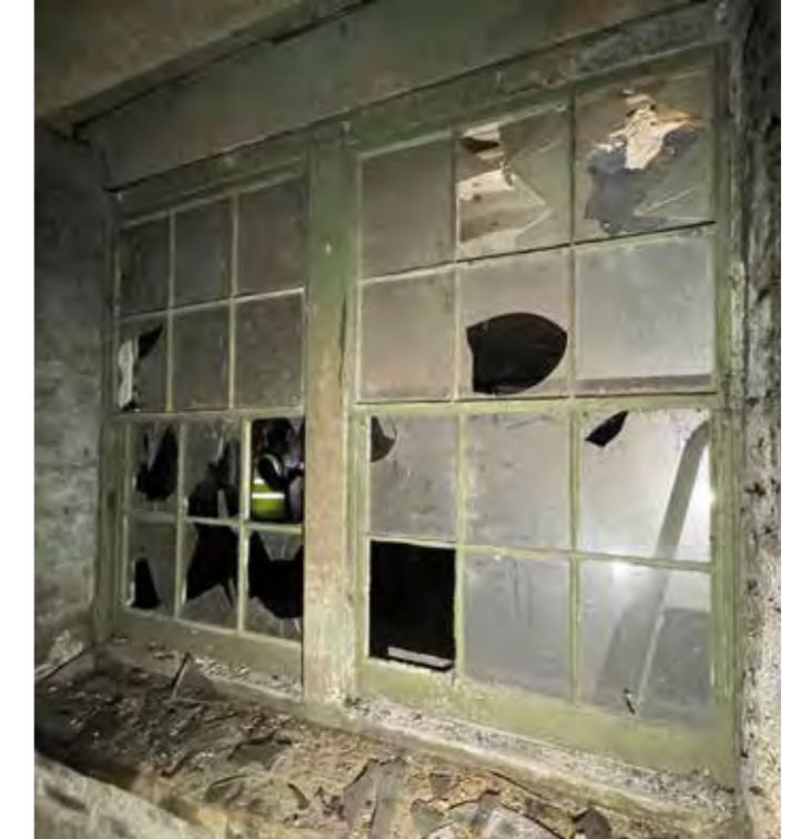
Historic sash window in need of repair
