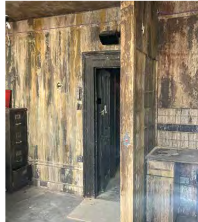
Historic skirting and picture rail. Doorcase with later modifications. Modern kitchenette. (35 NOST.)
