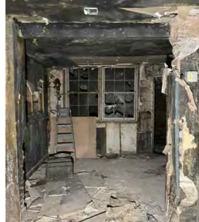
Modern joist supporting opening to front and back of basement. Boarded up fireplace possibly concealing range. Concrete screed.
