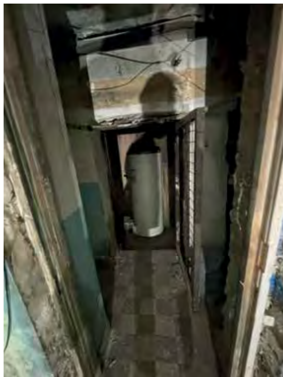
Coal vault in 11. Note tank
