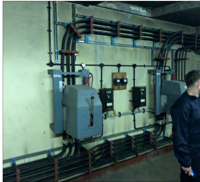
Existing Sub-station at basement level
