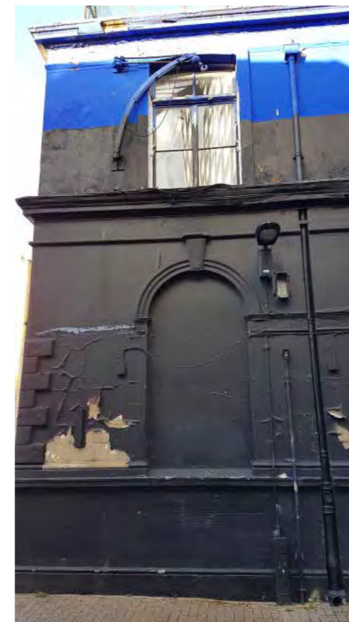
Existing wall crane
