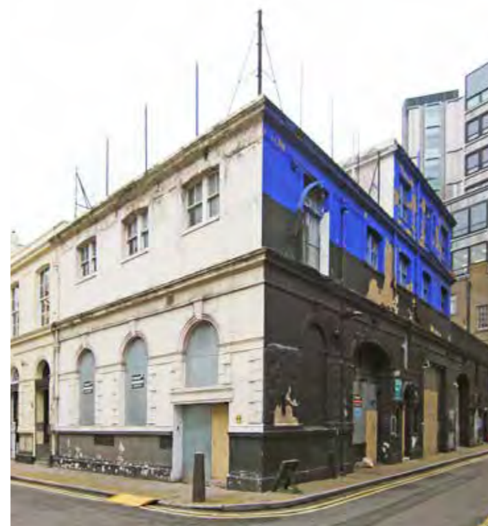
Existing Facade Condition as seen from West Central Street
