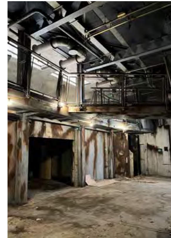
Existing ground floor condition 16A-18 West Central Street
