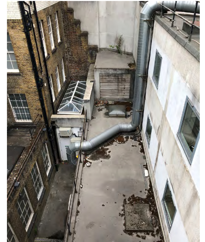
View 6: Existing lightwell between Selkirk House and the Embassy of Cuba highlights issues with overlooking
