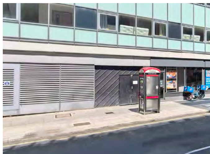
High Holborn elevation with ventilation louvres to existing UKPN substation and basement area
