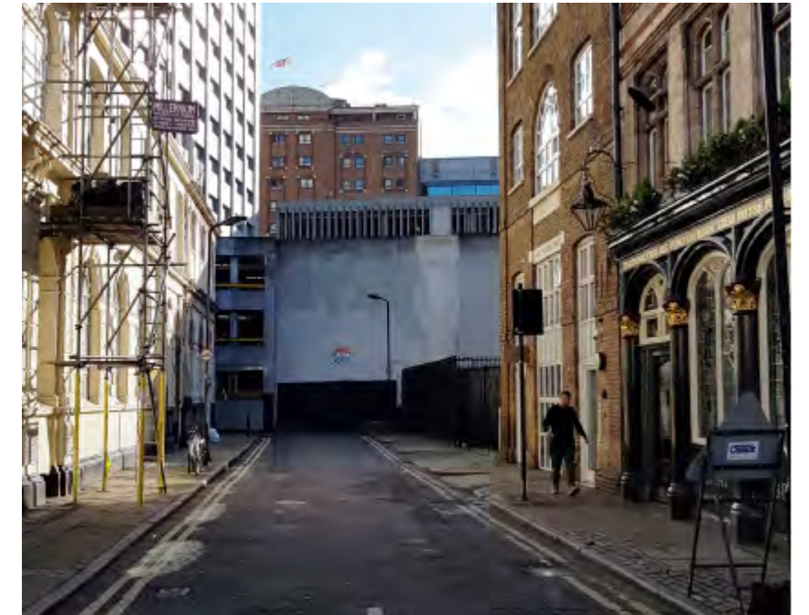
View 2: The Car Park ground floor condition is poorly activated and detracts significantly from the surrounding conservation areas. The lack of permeability at the building base leads to low levels of pedestrian traffic. The overall sense is one of neglect and discordance with surroundings.
