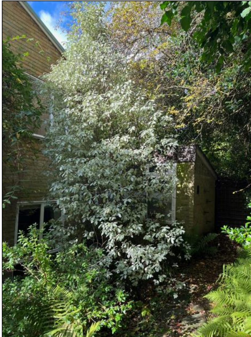
Photograph 1: Encroachment of structures
