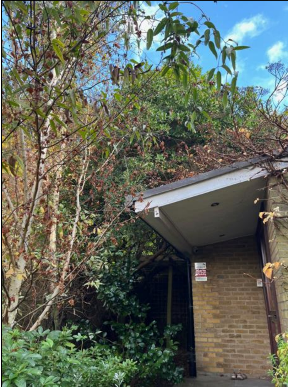
Photograph 3: T9 sprawling onto roof
