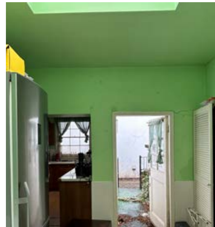
Figure 4.10 The ground floor pre-listing extension rear wall also showing signs of structural failure and dampness (see crack along the door lintel).
