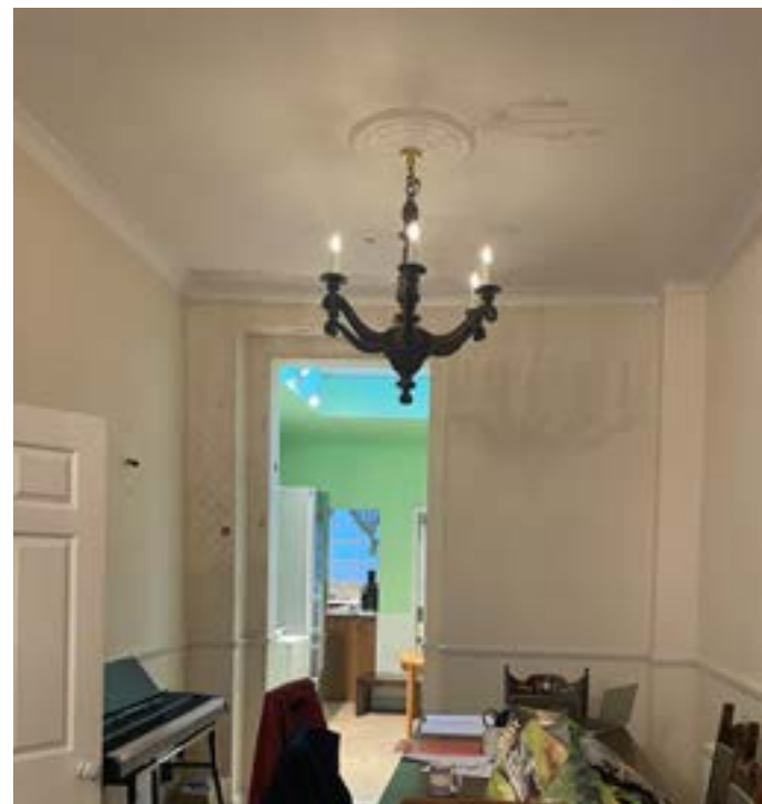
Figure 4.9 The ground floor original hall to the rear, showing signs of structural damage (see the bend to the rear wall) and dampness from the upstairs bathroom
