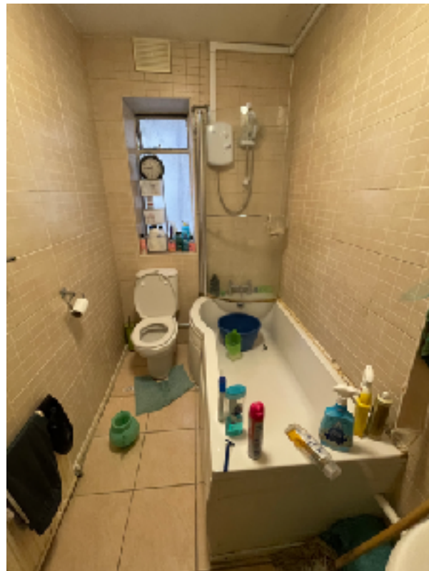
Passive vent above bathroom window
