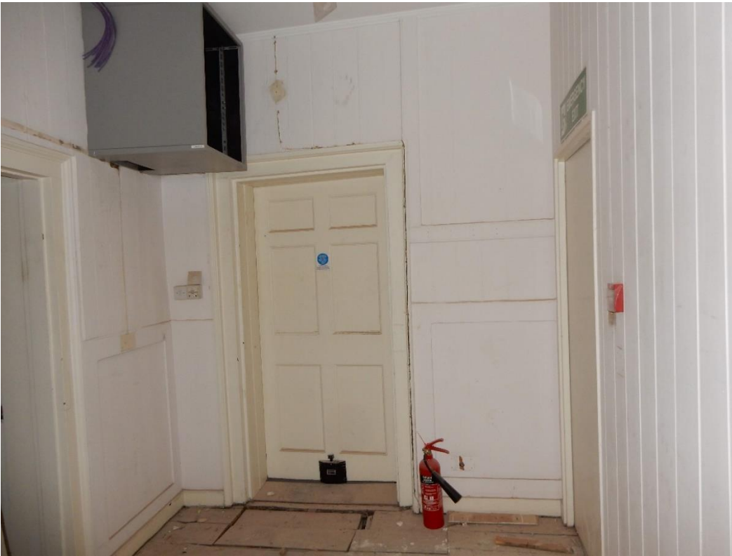
Existing Lobby partitioned off Stair Enclosure showing partition to be removed on right and door to be infilled on left. Door straight ahead will be entrance to Flat. Both doors to be removed are flush doors.
