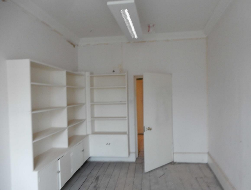
Office 5 looking south showing flush door to be infilled straight ahead and stud wall to left to be removed.
