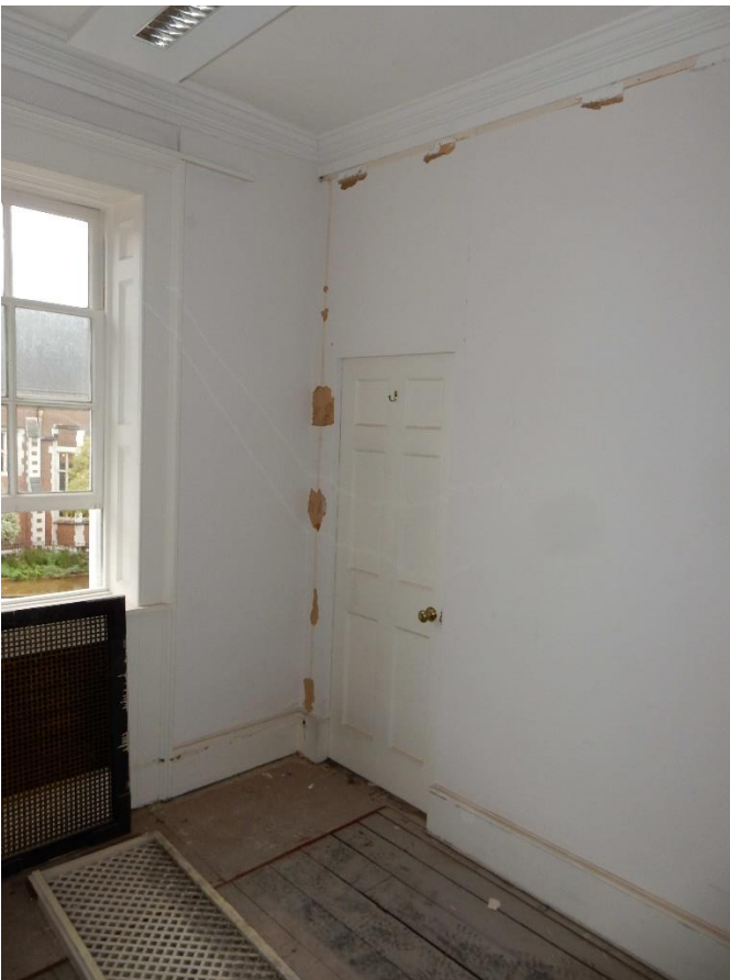
Office 5 looking north showing other end of wall to be removed on right
