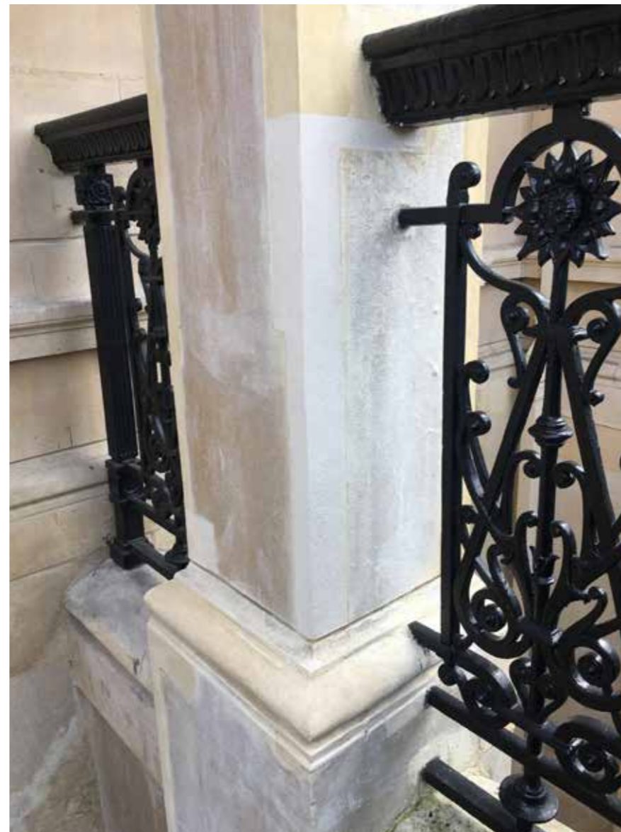
The corner repair after ten days on March 16. The side facing outwards is considered satisfactory, while the lateral face still has a strong contrast to the darker adjacent stone.
