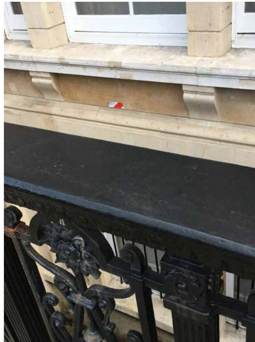
The repairs are almost imperceptible from the pavement which is the distance from which they are to be judged.
