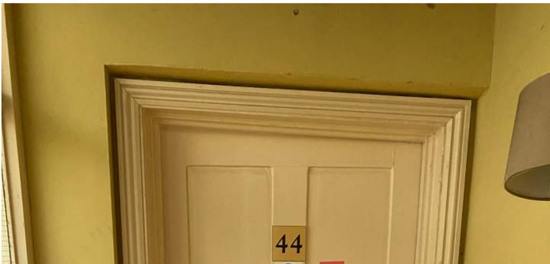
Fig 5: Examples of Deformed Partitions below Valley Beams
