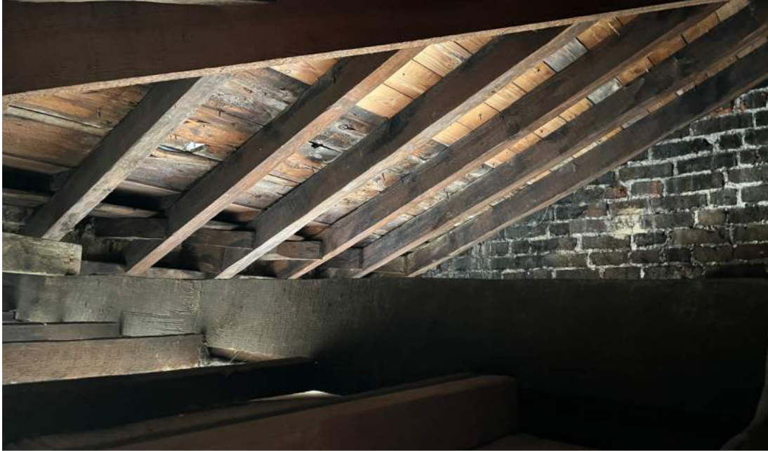
Fig 4: Inside of Roof showing Rafters, Hip Beam and Intermediate Ceiling Support Beam
