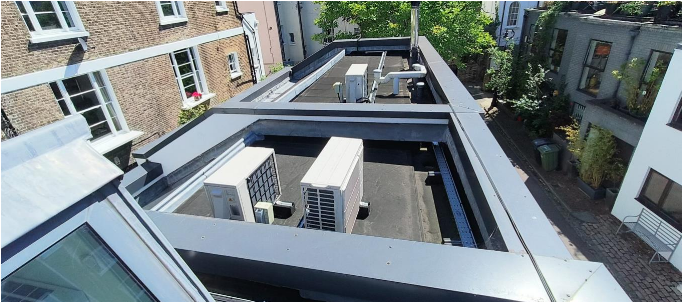
Figure 2 Photograph of the Condensers as Installed
