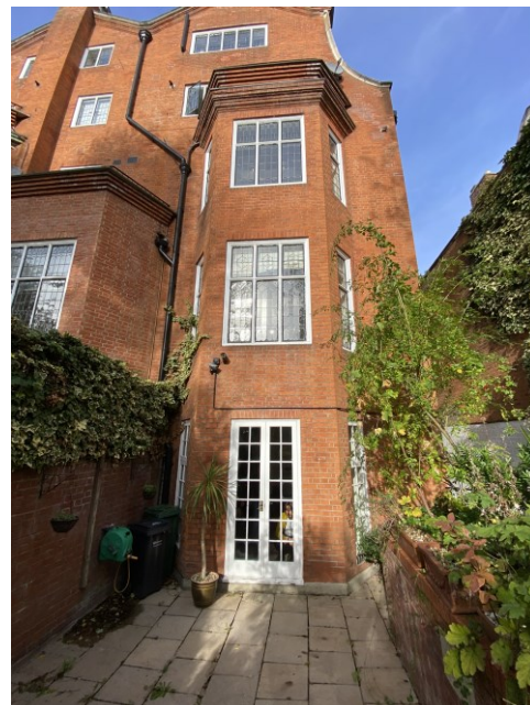
Figure 21 The existing patio area to the rear of Flat 1 and modern painted timber French doors.
