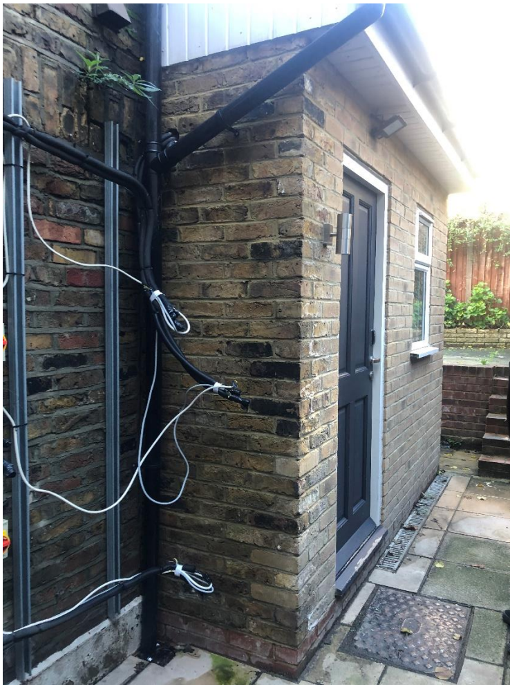
2. Side view of the rear extension to be retained and occupied by a kitchen.
