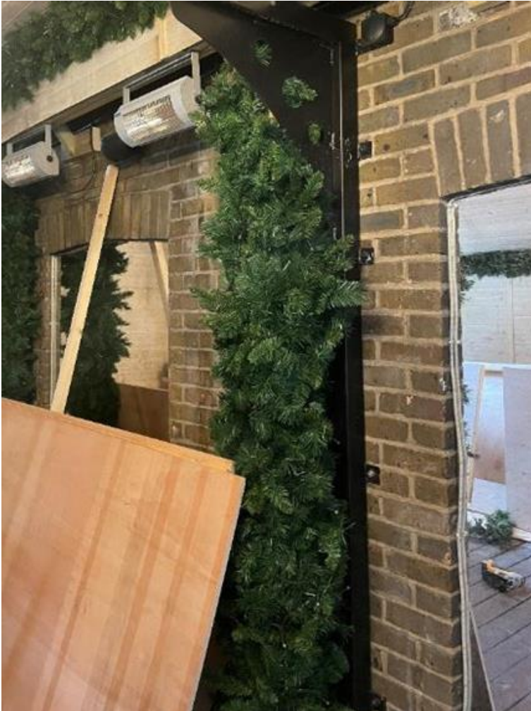
Plate 10: Brickwork of the building that the proposed structure will be fixed into.
