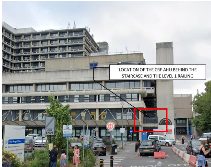
Image 10. View of CRF AHU, ducts and MRI-2, MRI-3 and MRI-4 quench pipes almost hidden behind the external staircase.
