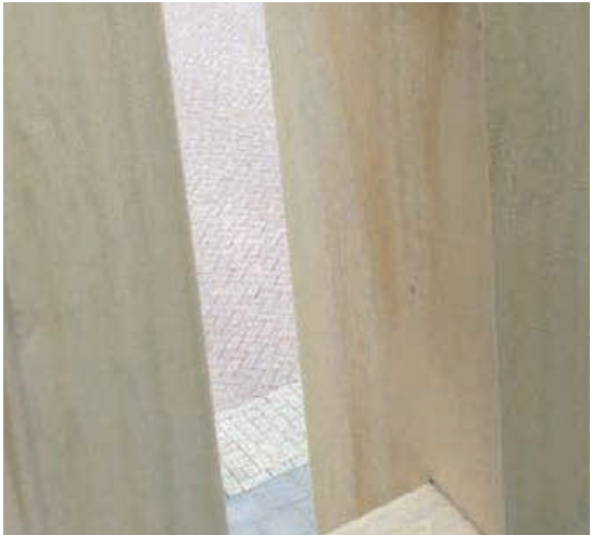
8.5 Reddish brown staining
