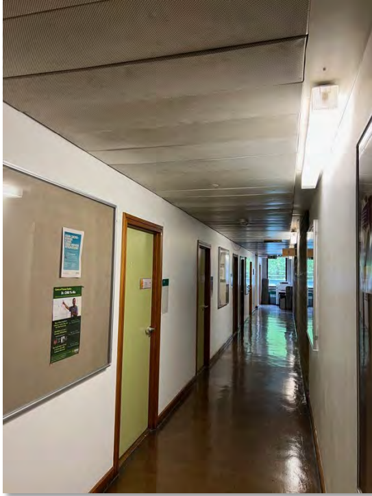
2 nd Floor Typical corridor view pre refurbishment Office/teaching room decorated flush panel doors with stained hardwood frames, architraves & skirtings
