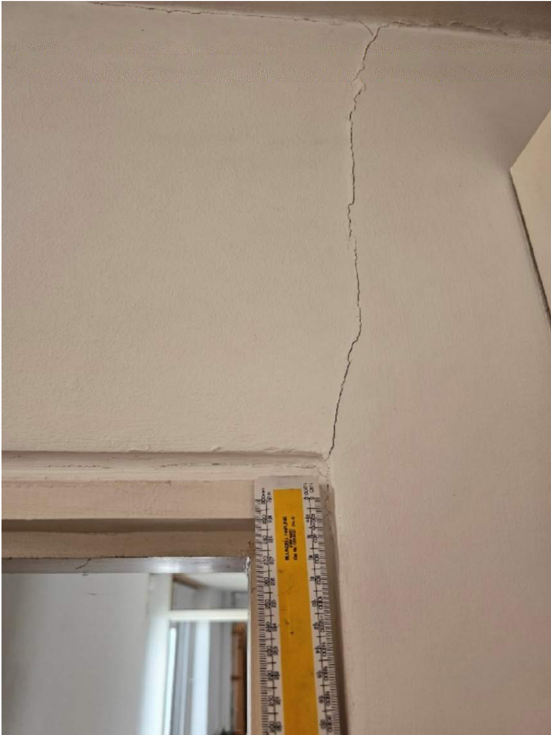
6 Photograph showing cracks in wall due to ongoing building movement
