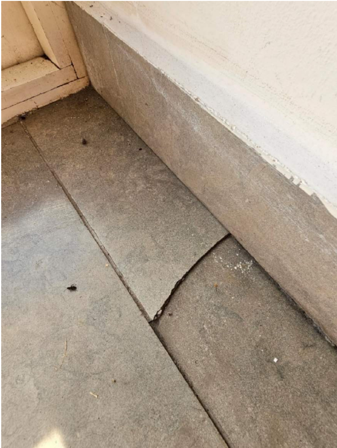
2 Photograph showing cracks in floor due to ongoing building movement
