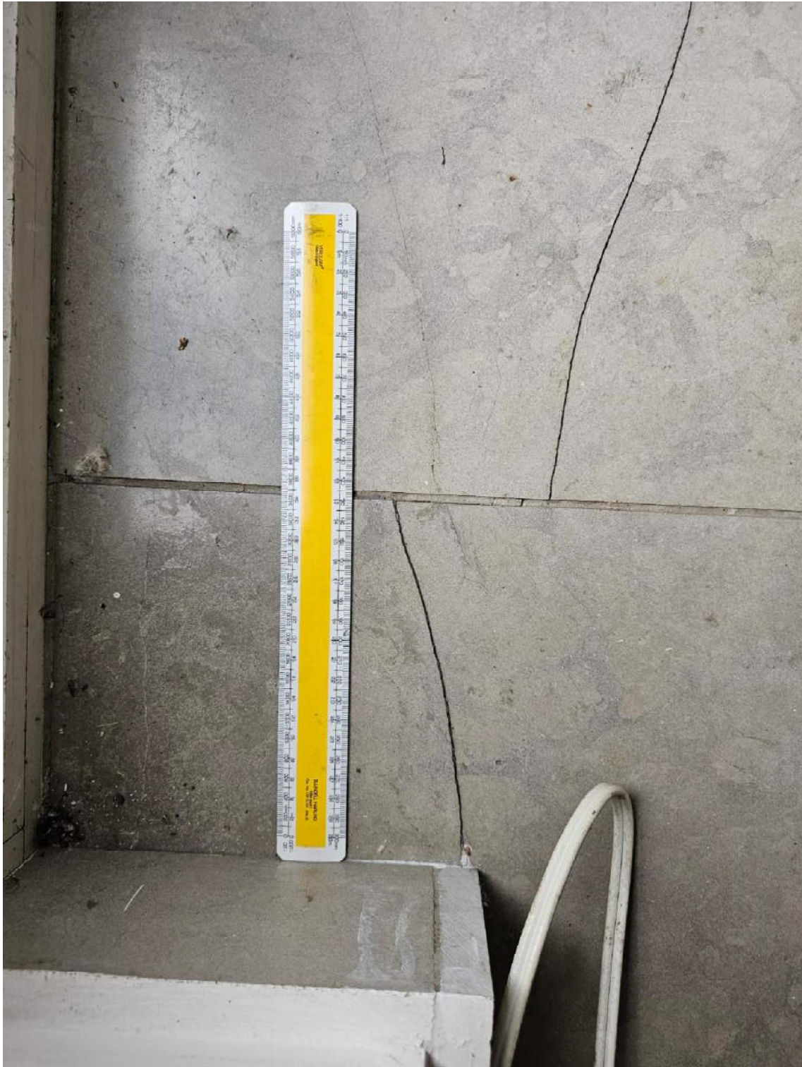
4 Photograph showing cracks in floor due to ongoing building movement
