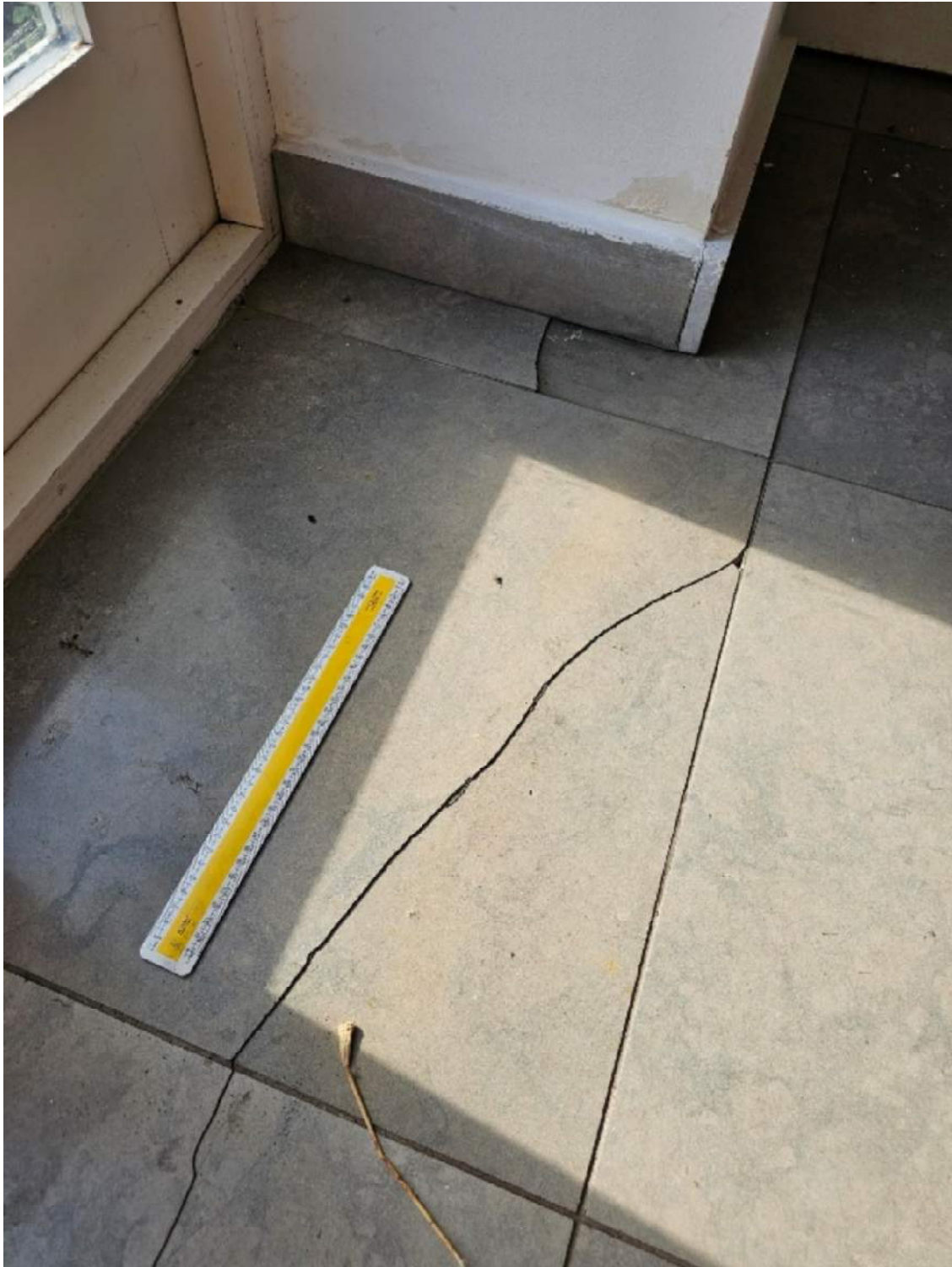
1 Photograph showing cracks in floor due to ongoing building movement
