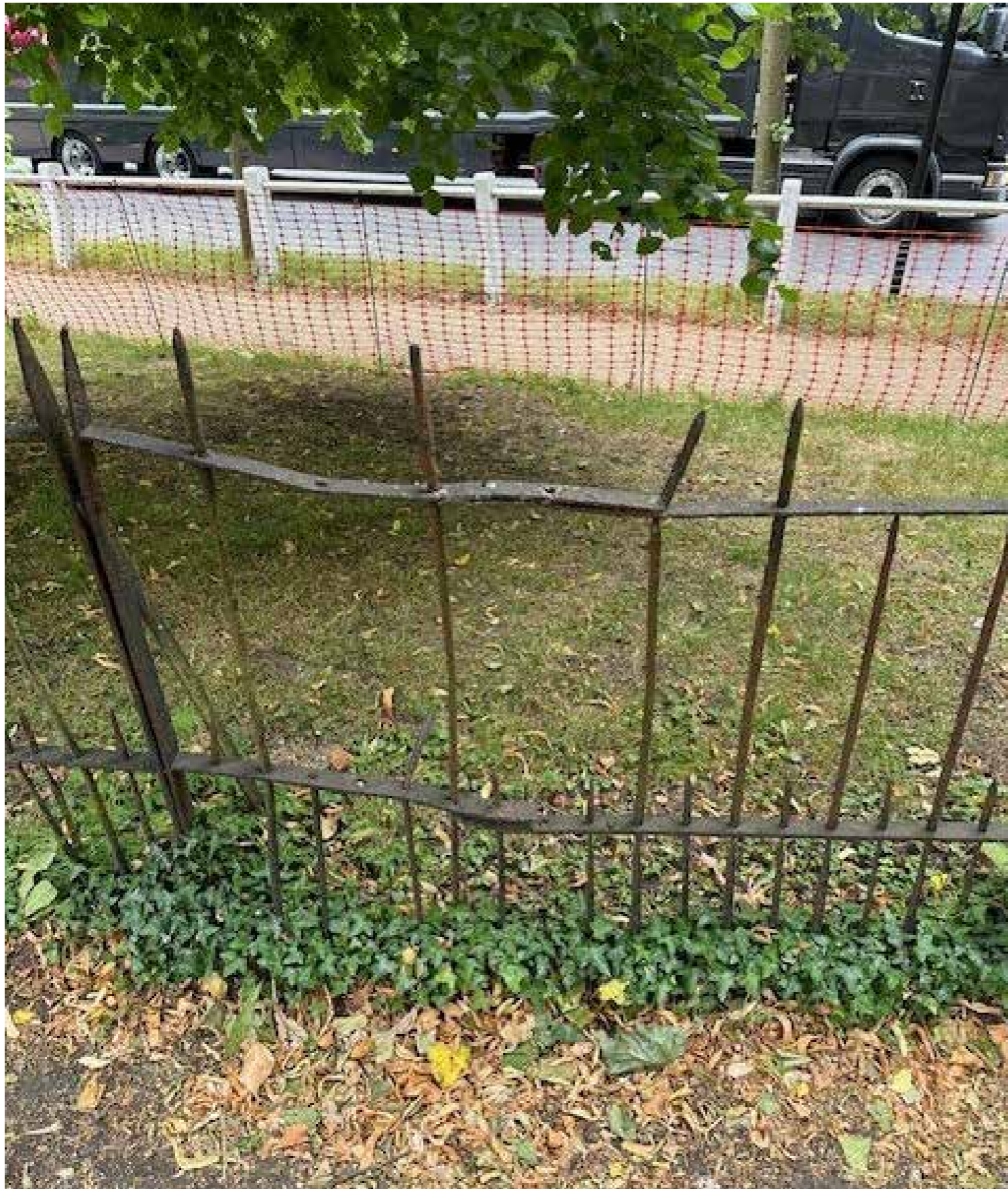
17. Panel Swith missing dog rails and upright
