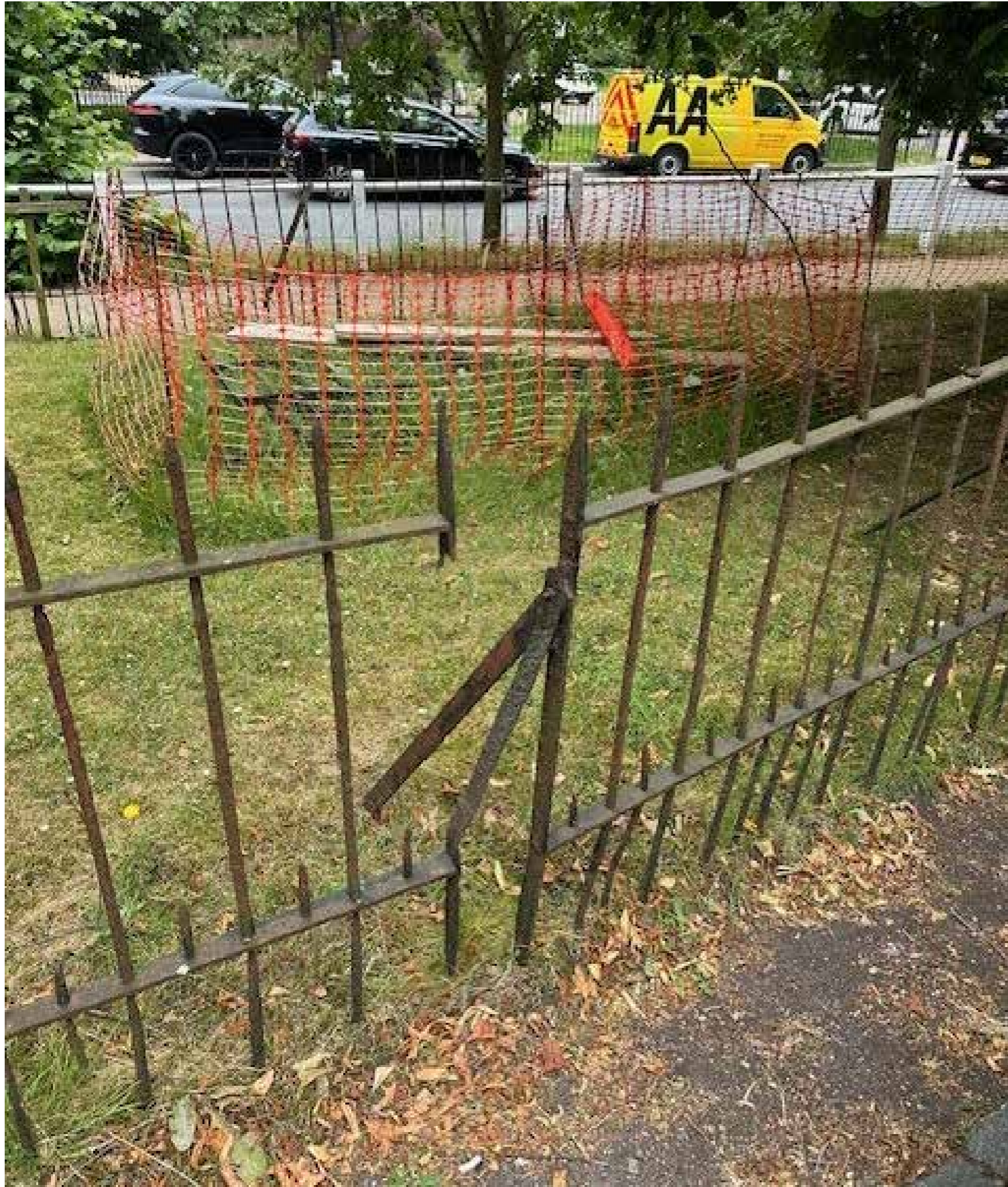
19. One panel missing end frame
