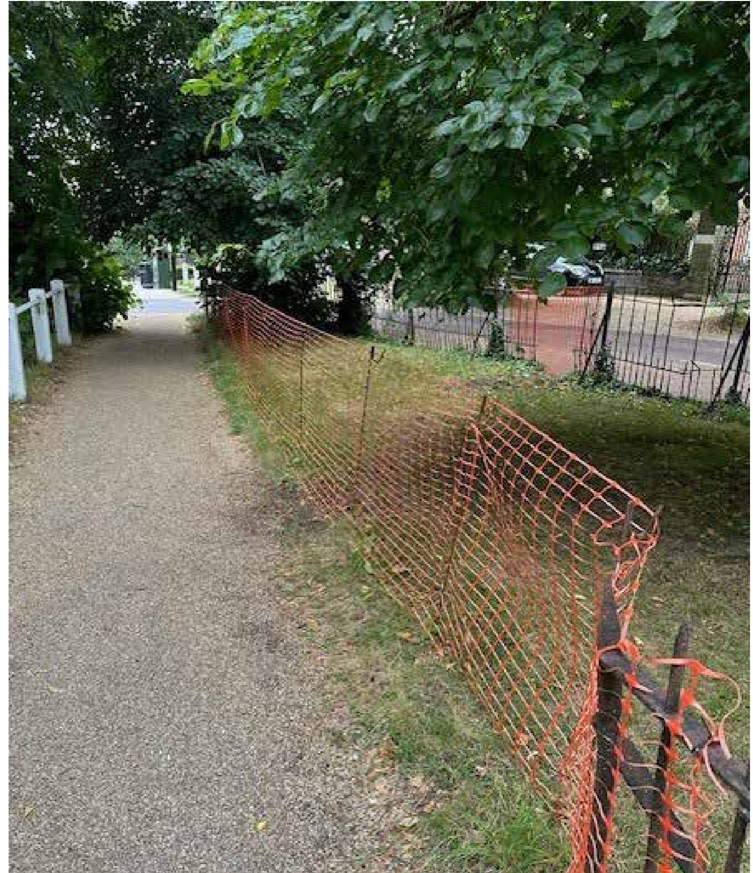
14. Extensive section of missing panels
