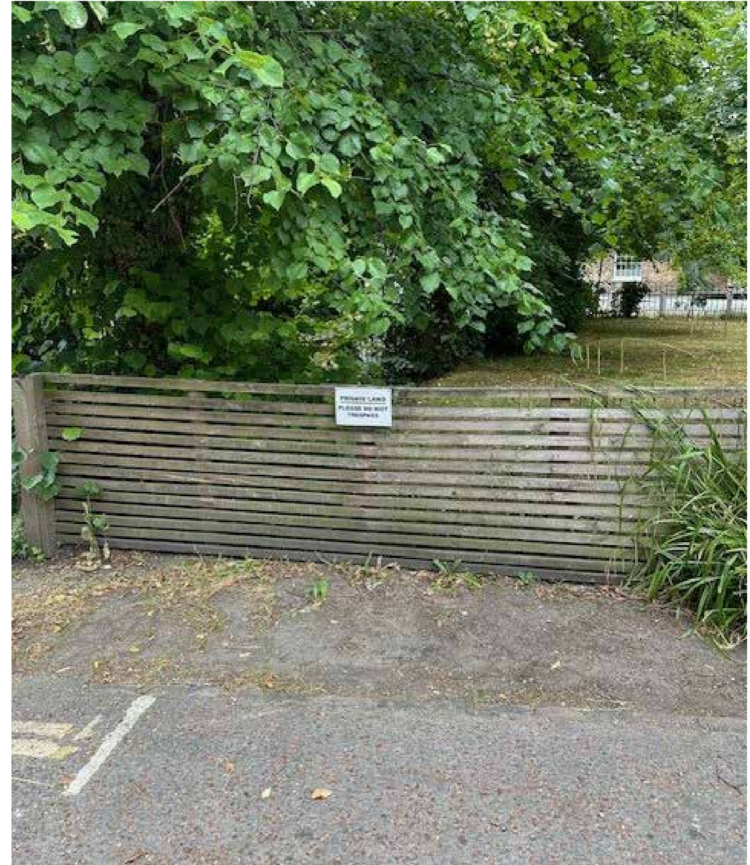
2. Circa. 4.4m length of panel missing (continued)
