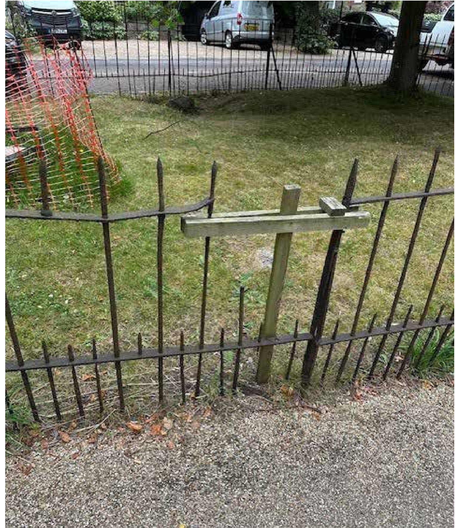
12. Broken panel (continued)
