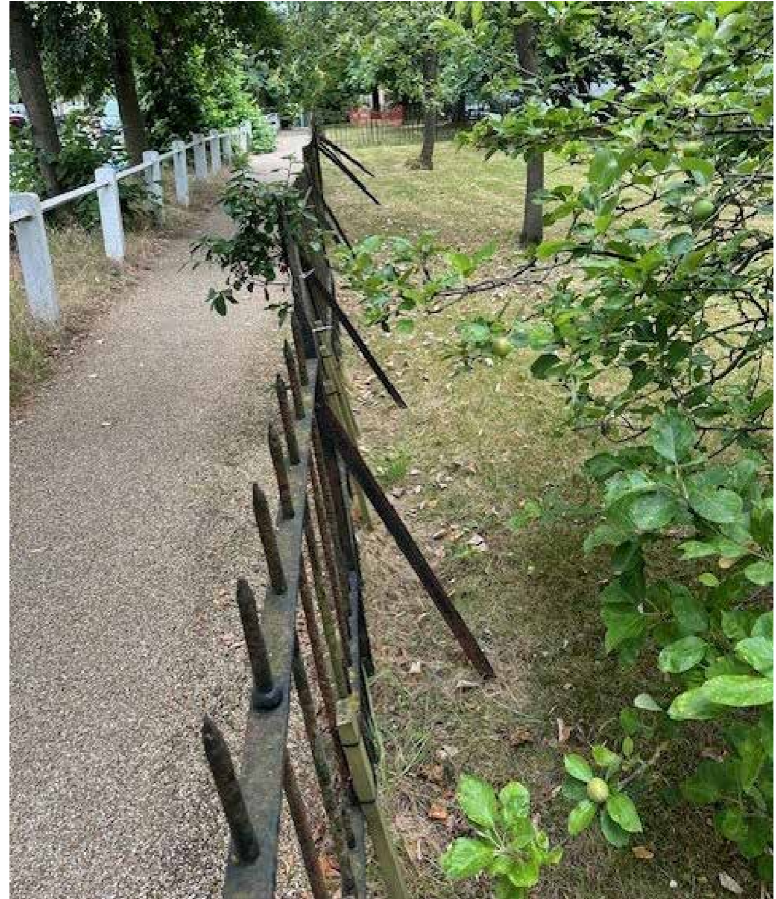
8. Remaining railings are bowed out and impede on to the adjacent footpath
