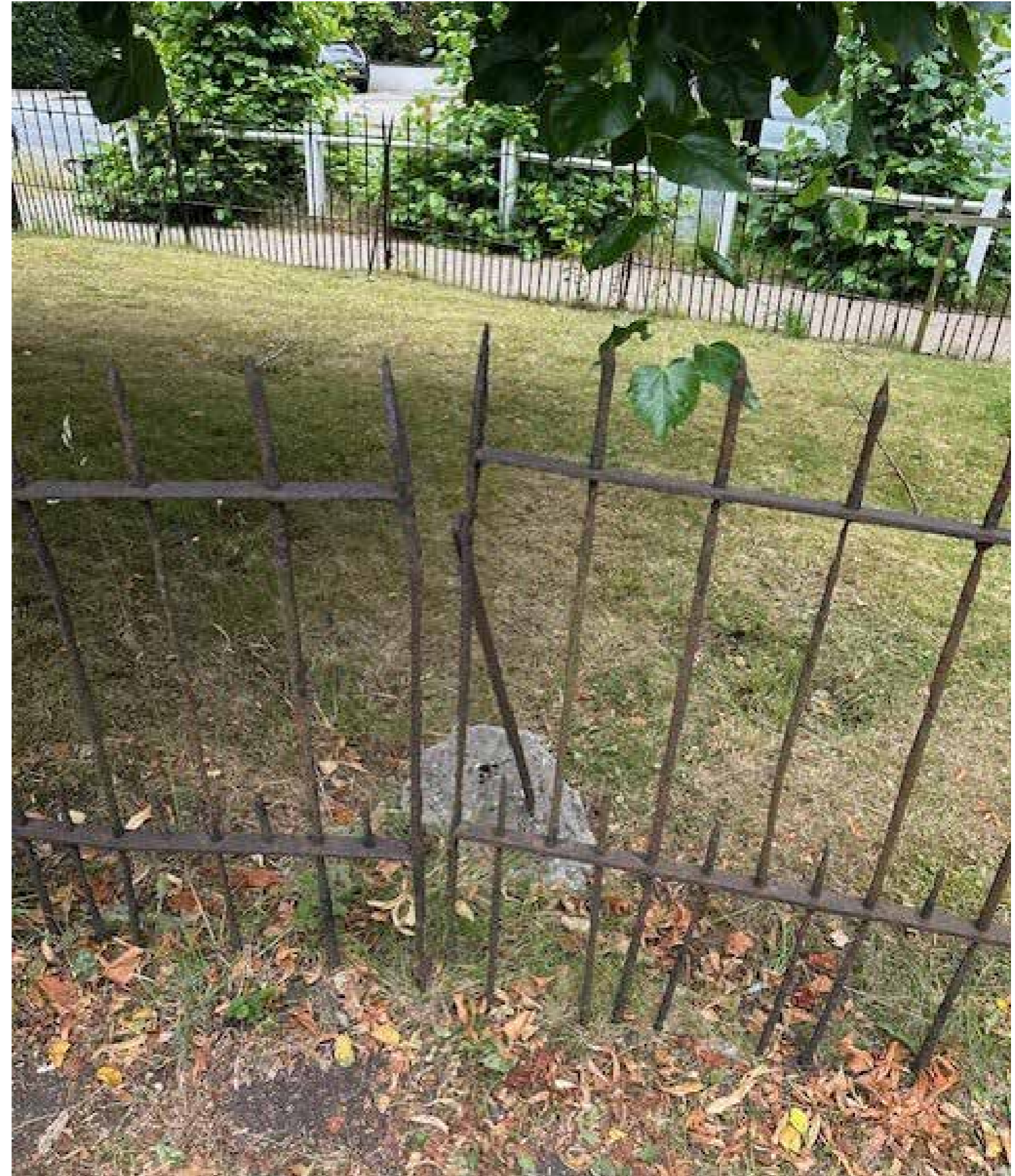
20. Broken connection between panels
